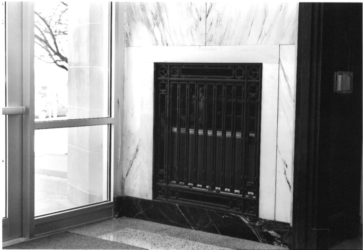
11. Kokomo High School recessed heat register in lobby
