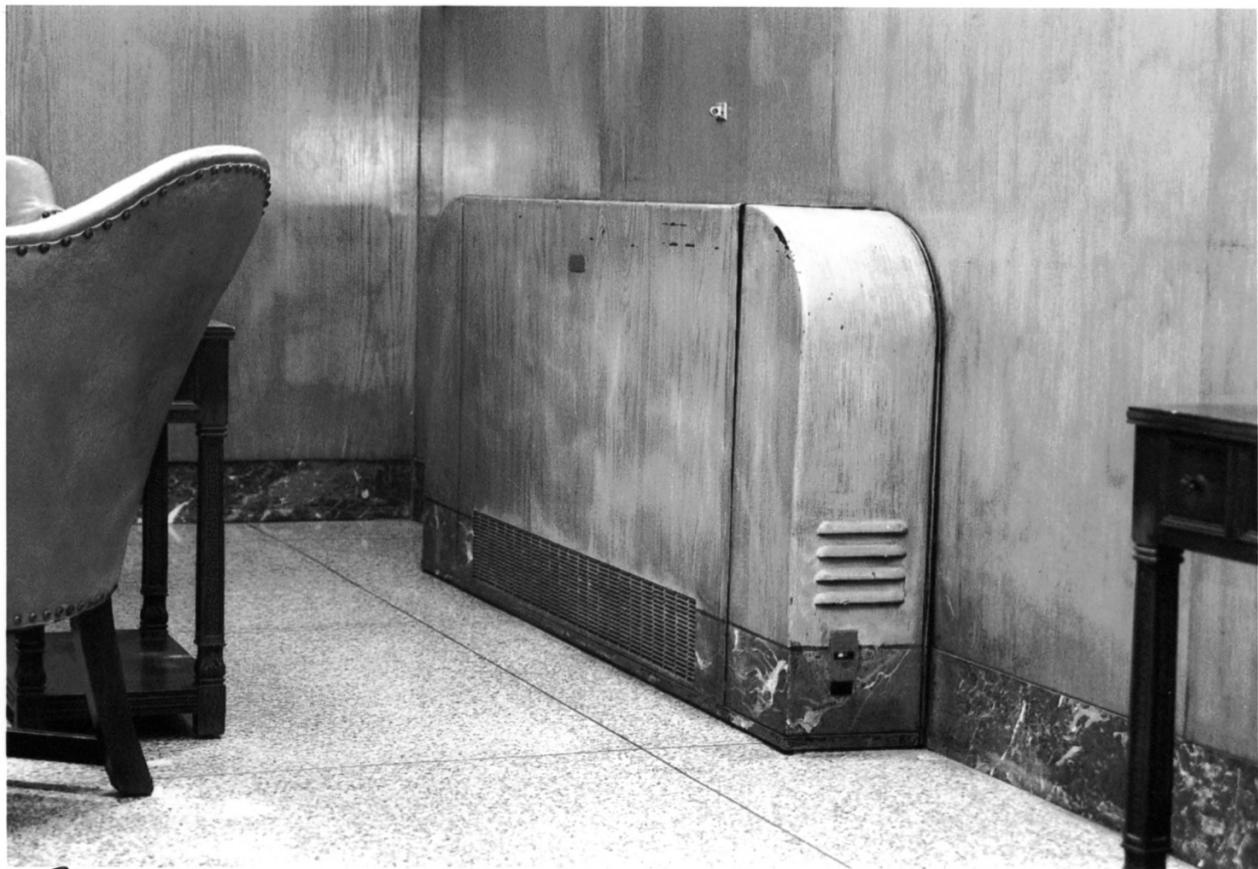
24. Faux Marble register, Memorial Room, Memorial Gym, Kokomo High Sch.
