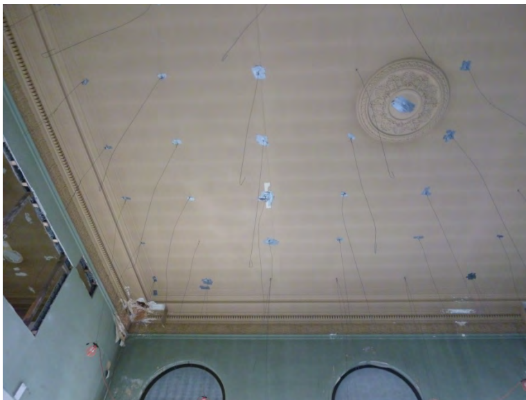
Figure 7: Looking at original ceiling in main banking hall during rehabilitation, following removal of suspended ceiling tiles during 2014 rehabilitation. Note decorative trim and medallion.
