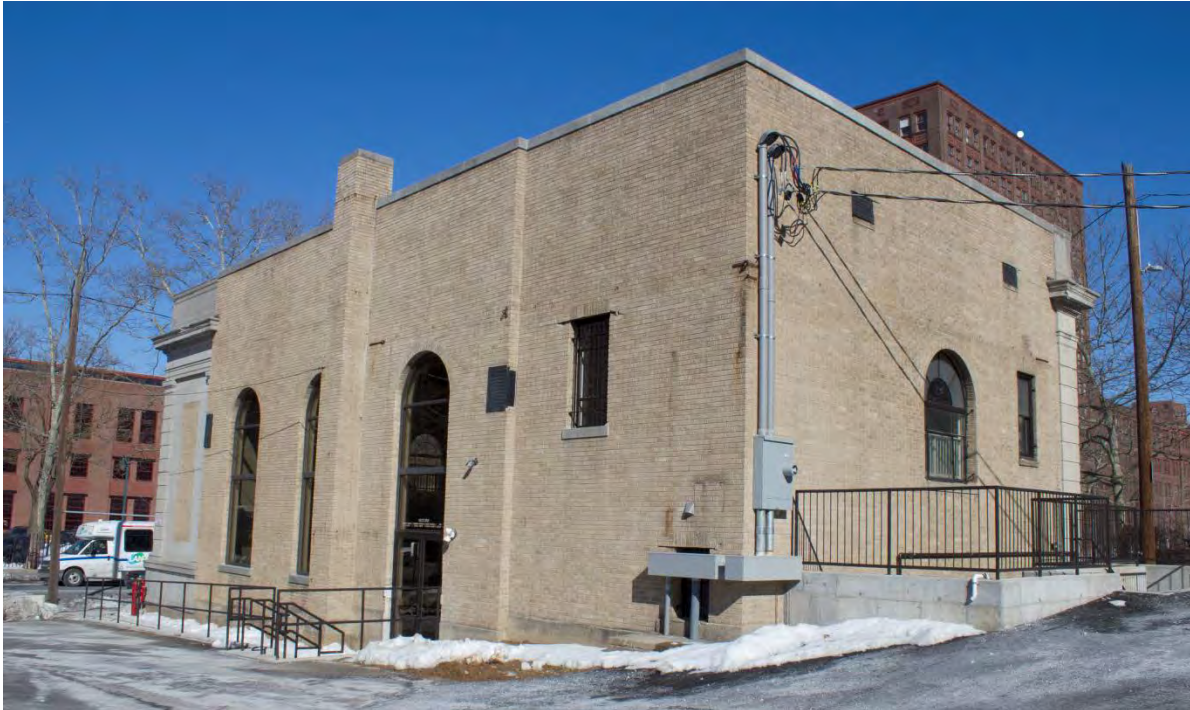
Photo 5—Rear and West elevations, facing NE, note conversion of window to accommodate new entrance into restaurant.
