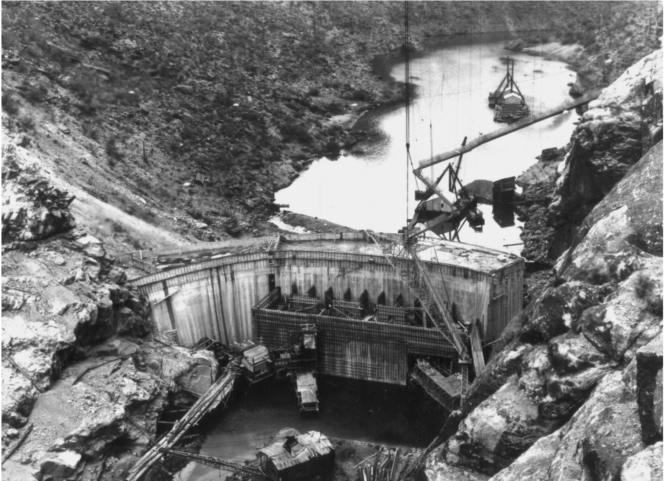
Historic Photo 5. Upstream view of the Horse Mesa Dam and power plant housing. Photo taken on October 2, 1926. Photo courtesy of the SRP.
