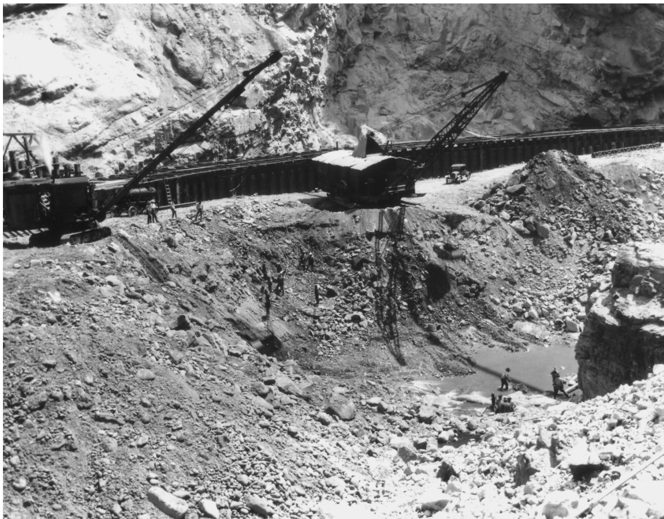
Historic Photo 2. View to the right (west side of the future Horse Mesa Dam showing excavation of the stream bed and the river diversion flume in background. Photo taken on April 1926. Photo courtesy of the SRP.
