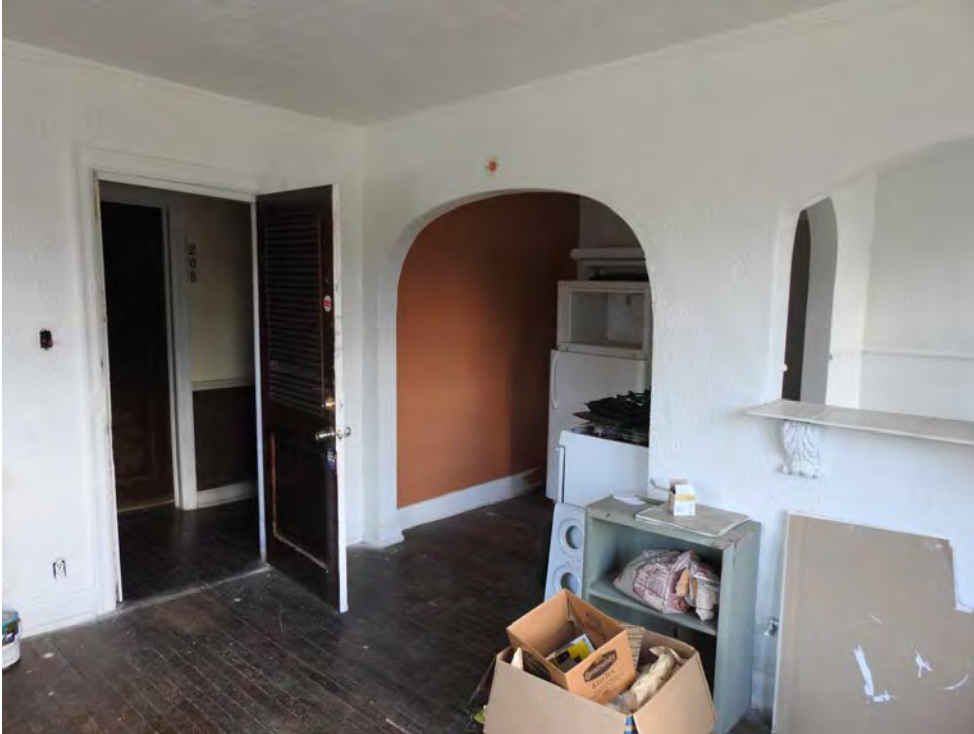
Photo 0009 – First floor apartment, typical, camera facing southeast. Arched entries are a characteristic to the building interior.
