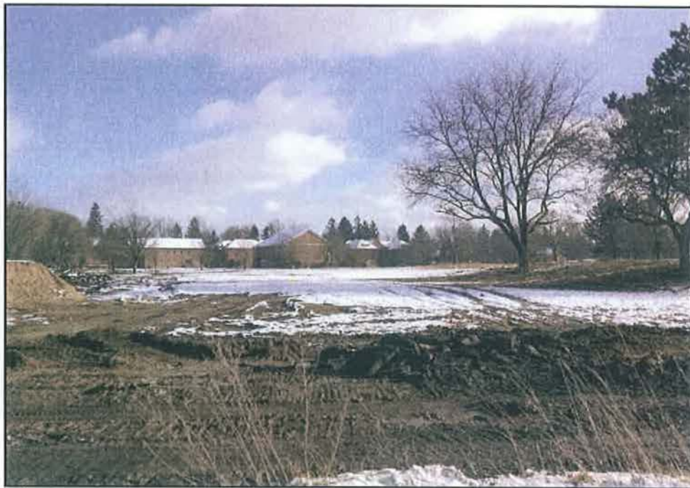
Figure 8. MPIIBS, Post MCP Demolition, View East from Former Intersection of Winding Lane and West Wind Drive
