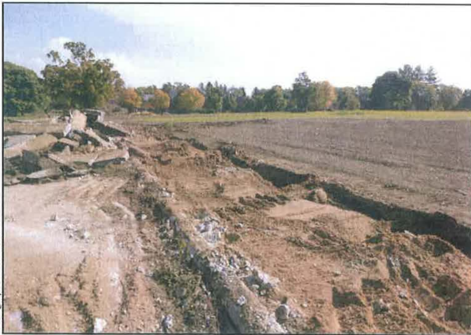
Figure 7. Sidewalk Removal and Landscape Restoration, North of Former Parking Lot, View East toward MPIIBS
