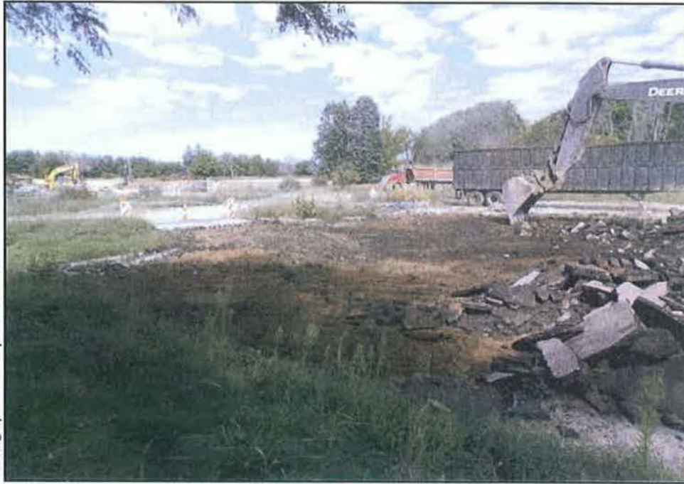
Figure 4. Parking Lot Removal at Southeast Corner of West Wind and Winding Lane, West Half, View North
