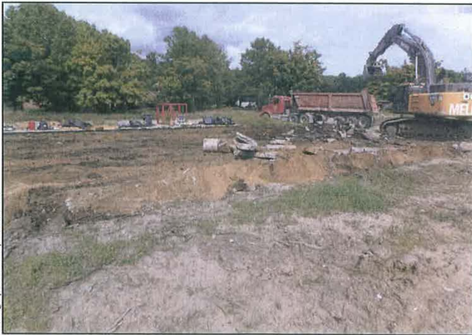
Figure 5. Parking Lot Removal at Southeast Corner of West Wind and Winding Lane, View Northeast
