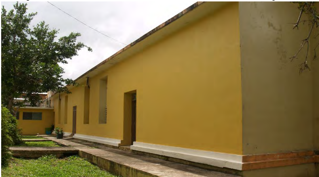
Figure 5. Building's rear, with the 1950's concrete bathroom annexed at the southern wing's rear.
