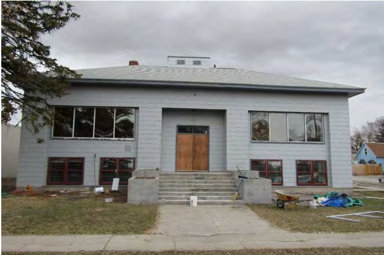
Valley Masonic Lodge No. 21, detail of west façade, view to east. MT_BroadwaterCounty_ValleyMasonicLodgeNo21_0009.
