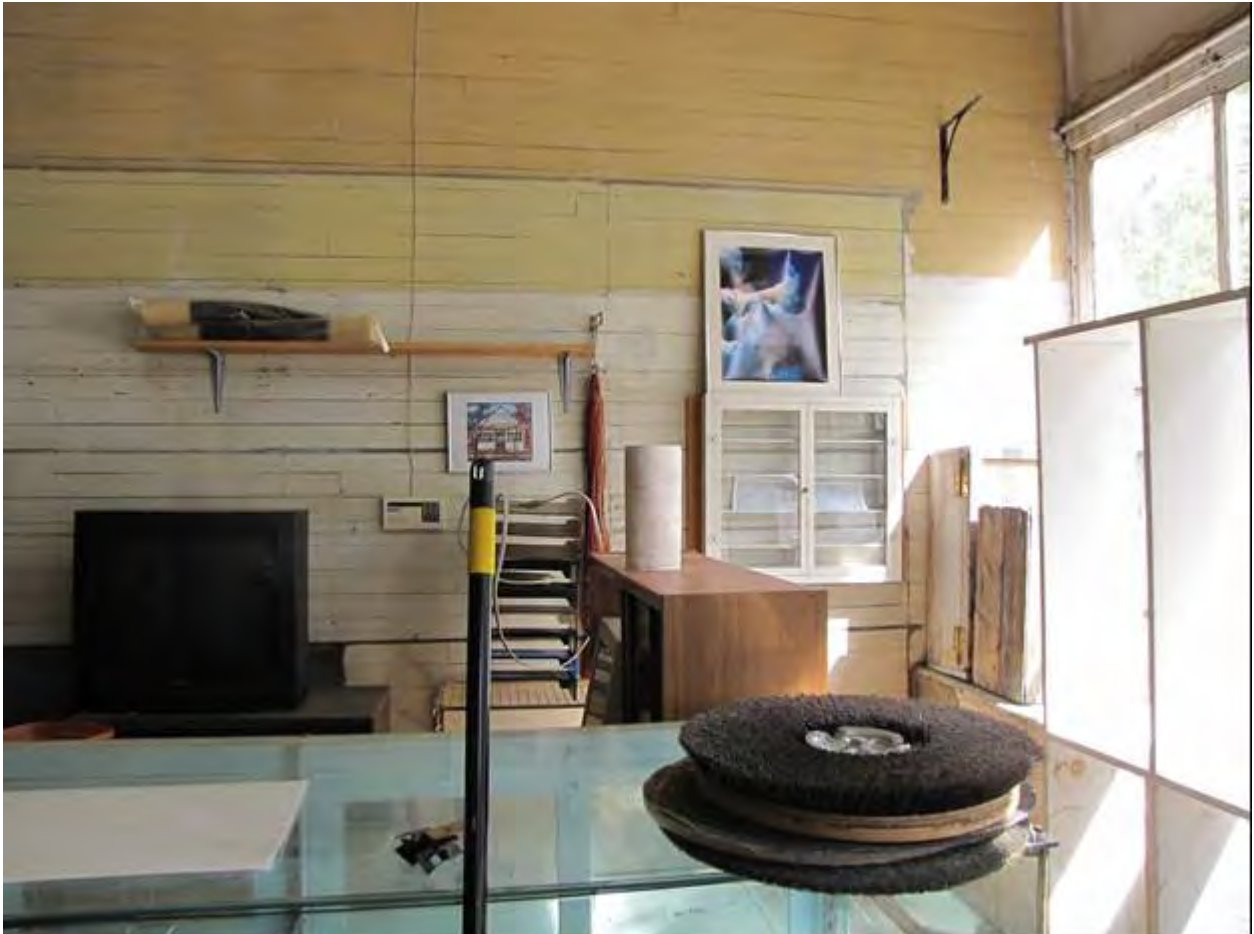
MT_LewisAndClarkCounty_DorseyGroceryAndResidence_0013. Grocery, interior, east wall with silhouette of original shelving, view to E.
