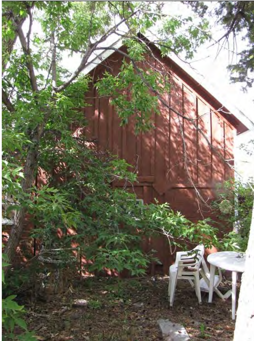
MT_LewisAndClarkCounty_DorseyGroceryAndResidence_0024. Garage/Carriage House, south wall of carriage house component, view to N.
