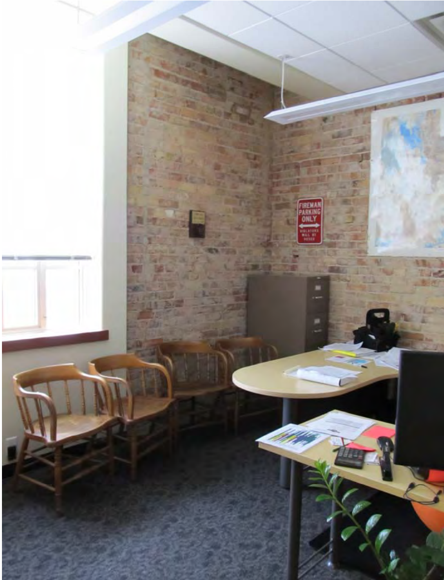
Photo 20 of 21: Building Department office, showing typical exterior wall treatment and bulkhead detail at edge of ceiling. Camera facing southeast. December 22, 2014. (Anya Grahn)
