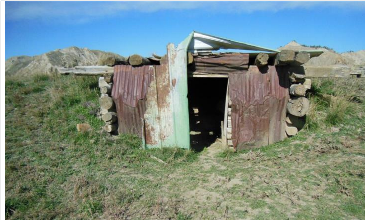
MT_Blaine County_Ervin Homestead/GistBottom_HD_0039 Gist Dugout Shed #1. South elevation. View to the north.
