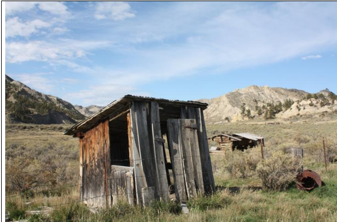
MT_Blaine County_Ervin Homestead/GistBottom_HD_0033 Gist Frame Shed. South and east elevation. View to the northwest.
