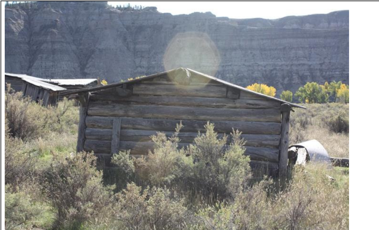
MT_Blaine County_Ervin Homestead/GistBottom_HD_0037 Gist Log Shop. North elevation. View to the south.
