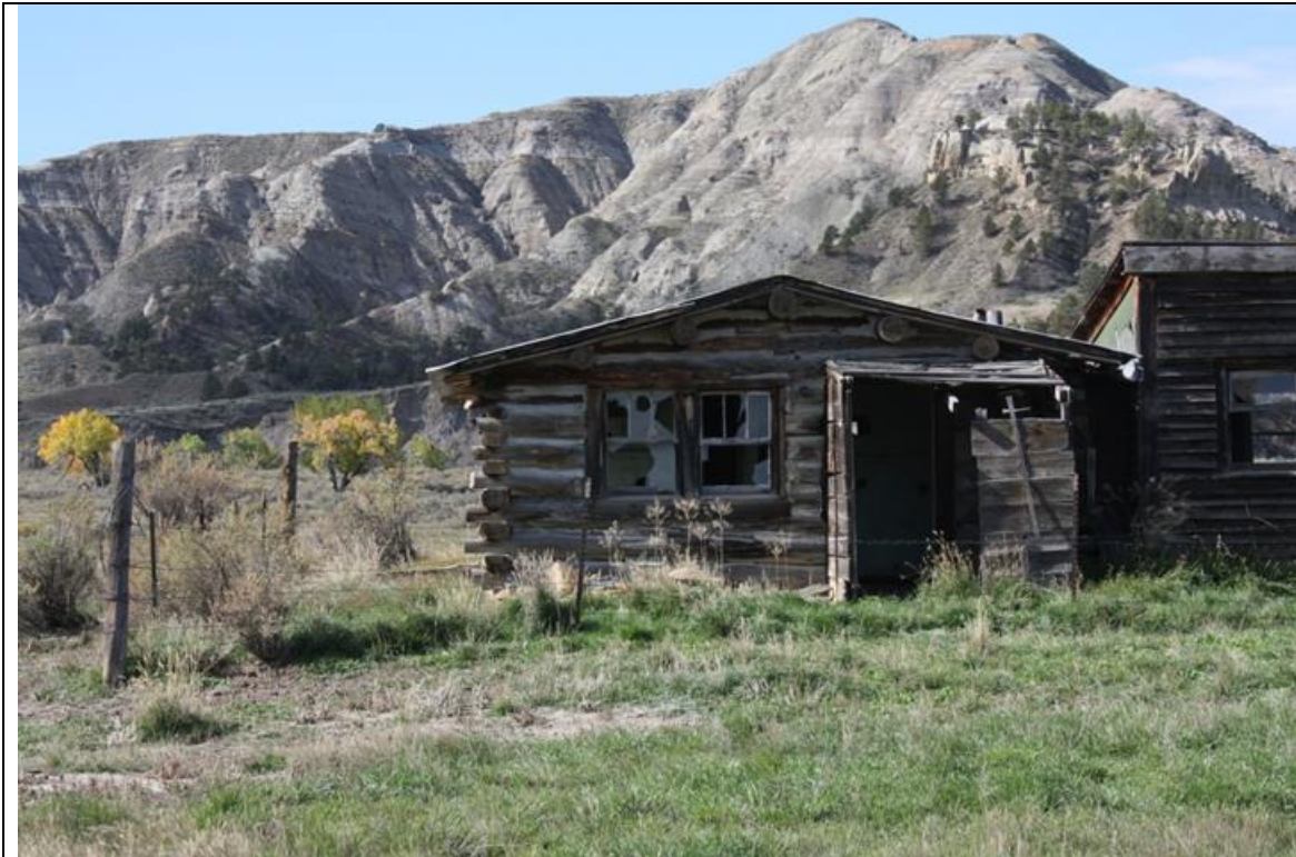
MT_Blaine County_Ervin Homestead/GistBottom_HD_0024 Gist Residence. Detail of south wing. East elevation. View to the west.
