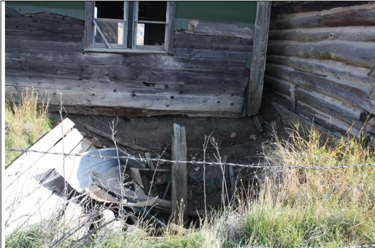
MT_Blain County_Ervin Homestead/GistBottom_HD_0028 Gist Residence. Detail of collapsed well, west elevation. View to the east.
