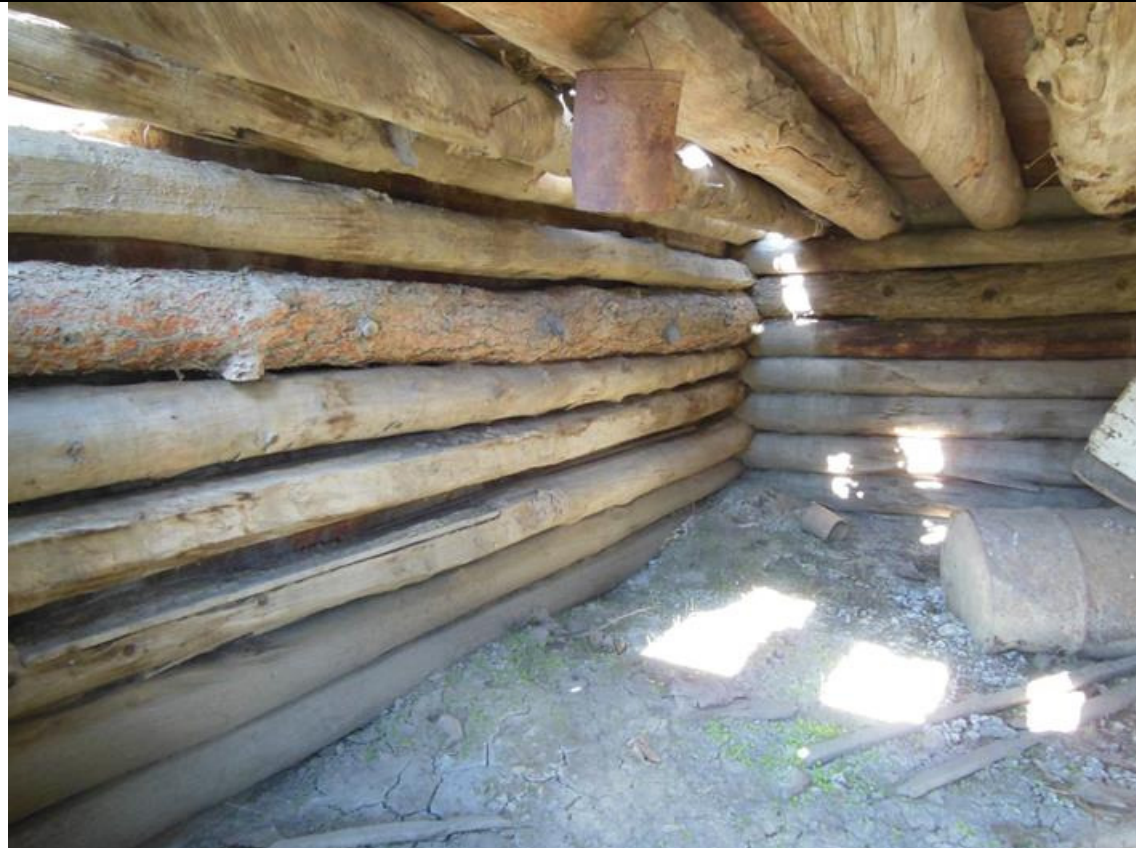
MT_Blaine County_Ervin Homestead/GistBottom_HD_0042 Gist Dugout Shed #1. Interior west wall. View to the north.
