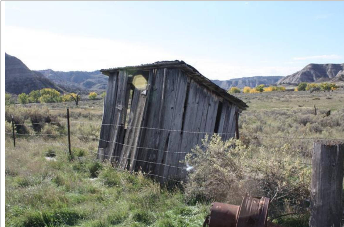
MT_Blaine County_Ervin Homestead/GistBottom_HD_0034 Gist Frame Shed. East and north elevation. View to the southwest.
