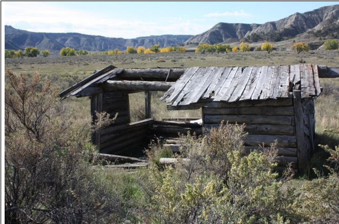
MT_Blaine County_Ervin Homestead/GistBottom_HD_0038 Gist Log shop. East elevation. View to the west.
