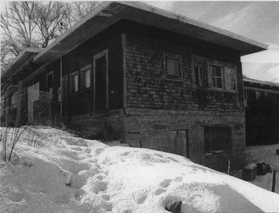
Photo 0012. East elevation showing north extension. Montana, Wyoming & Southern Railroad Depot. View to the southwest.
