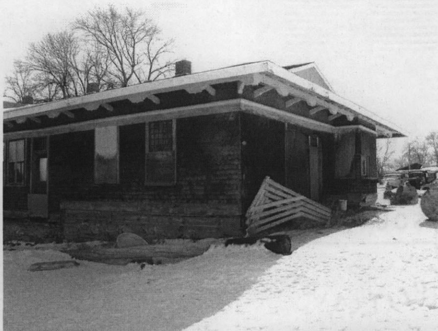
Photo 0017. North façade and west elevation of the Montana, Wyoming & Southern Railroad Depot. View to the south-southeast.
