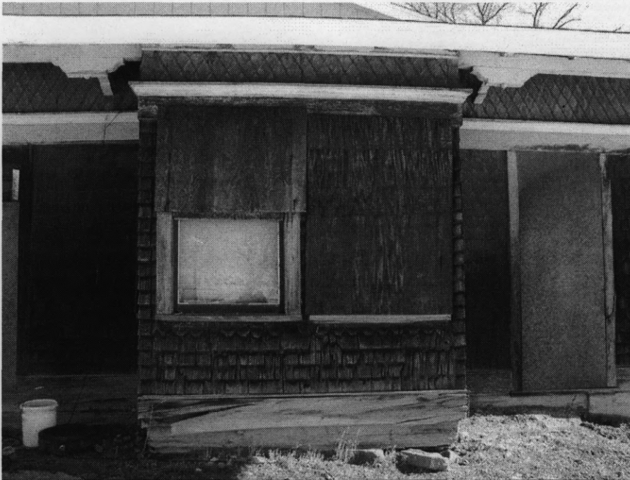
Photo 0019. Detail of ticket booth of Montana, Wyoming & Southern Railroad Depot. West elevation. View to the east.
