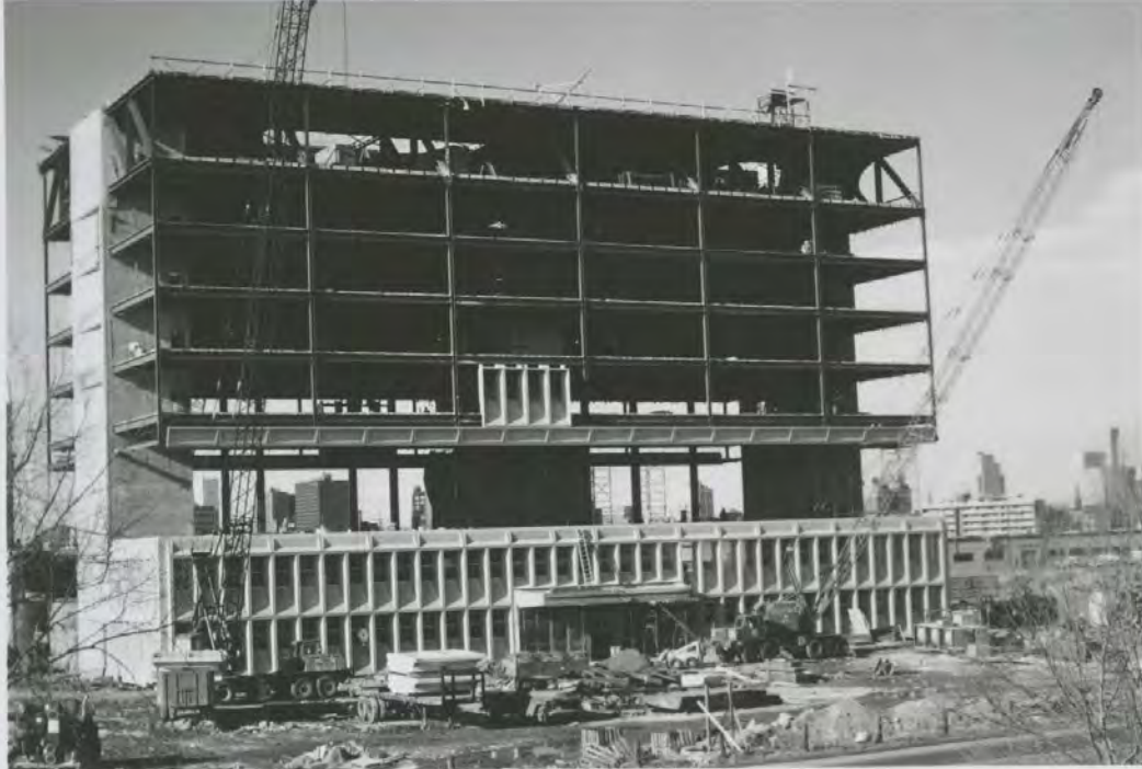
Figure 5: Construction photograph of the Armstrong Rubber Company Building, view towards east elevation, 1969 (Source: Marcel Breuer Digital Archive, Syracuse University Libraries 2018)
