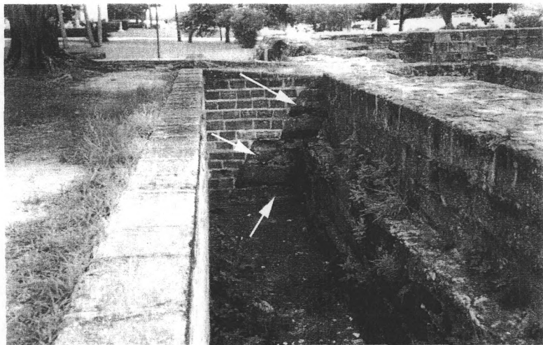
Figure 8. View of west wall profile of the coquina ruins at Old Fort Park, facing north, showing different construction episodes. Lowest arrow points to the first (original) episode of construction with the Hull addition above it and the WPA restoration on top.
