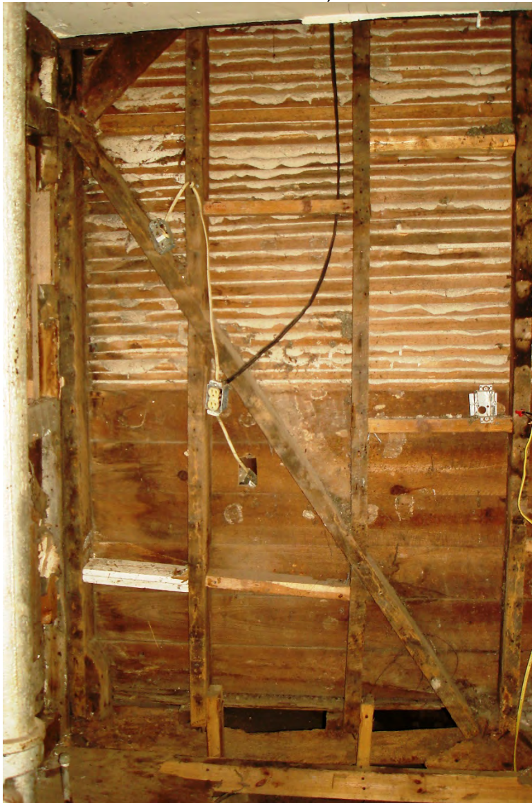
12 of 17: Room 101, interior framing of the east wall. (Photo taken in 2012, before the rear additions were removed.)
