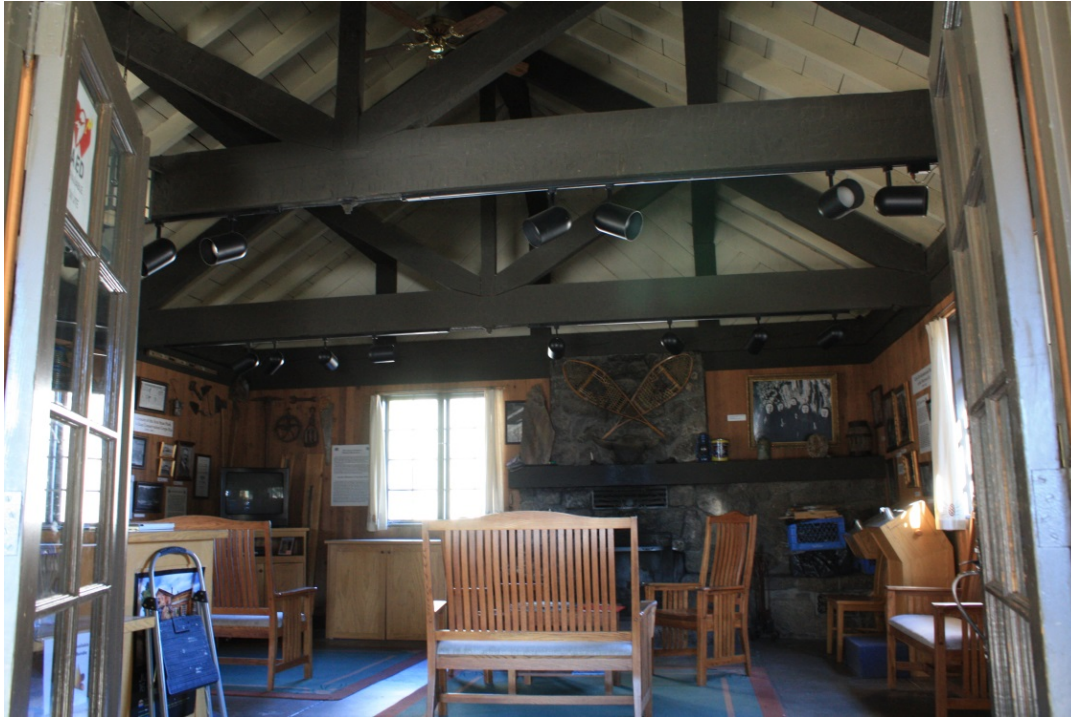
MT_JeffersonCounty_Lewis&ClarkCavernsHD_0013: Feature 6, Interior of Headquarters through entrance, with original furnishings, fireplace, open trusses.
