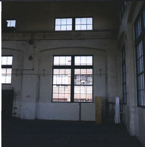
Nisqually Power Substation, Pierce County, WA West Interior Wall, Typical Window Set, Main Floor 09/00, M. Sullivan, Photo
