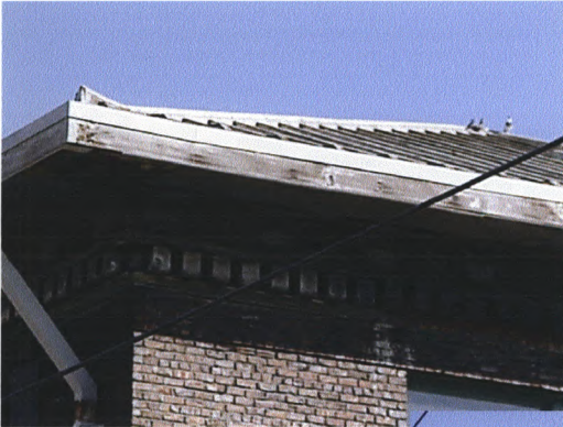
Nisqually Power Substation, Pierce County, WA Detail: Roof/Cornice Dentil, Southwest Corner, Looking Northeast 09/00, M.Sullivan, Photo
