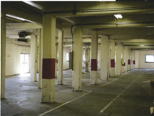
Nisqually Power Substation, Pierce County, WA Interior Detail, First Floor, Look- ing South 09/00, M.Sullivan, Photo
