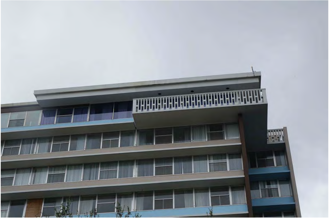
Photo 16 West wing 11 th floor balcony, facing south Photographed by Gregory Smith, October 2015
