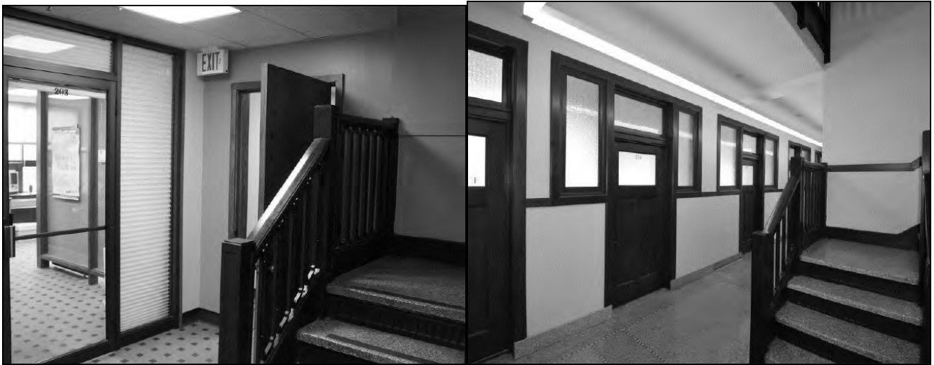
Figures 33-34: second floor hall intersection, looking northeast, 2014 (left), 2016 (right) (photos courtesy of Neumann Monson Architects, Iowa City, right)
