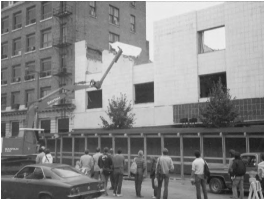
Figure 20: Demolition of the fire-damaged building to the south, 1983 (Courtesy Neumann Monson Architects)
