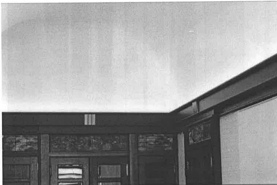
Detail of cove lighting in arcade
