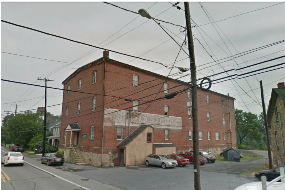
United Cigar Company/General Cigar Company Tobacco Warehouse (ca. 1910), Main Street, Salunga. Note the replacement windows and altered entrances (Source: Google Earth, July 2013).
