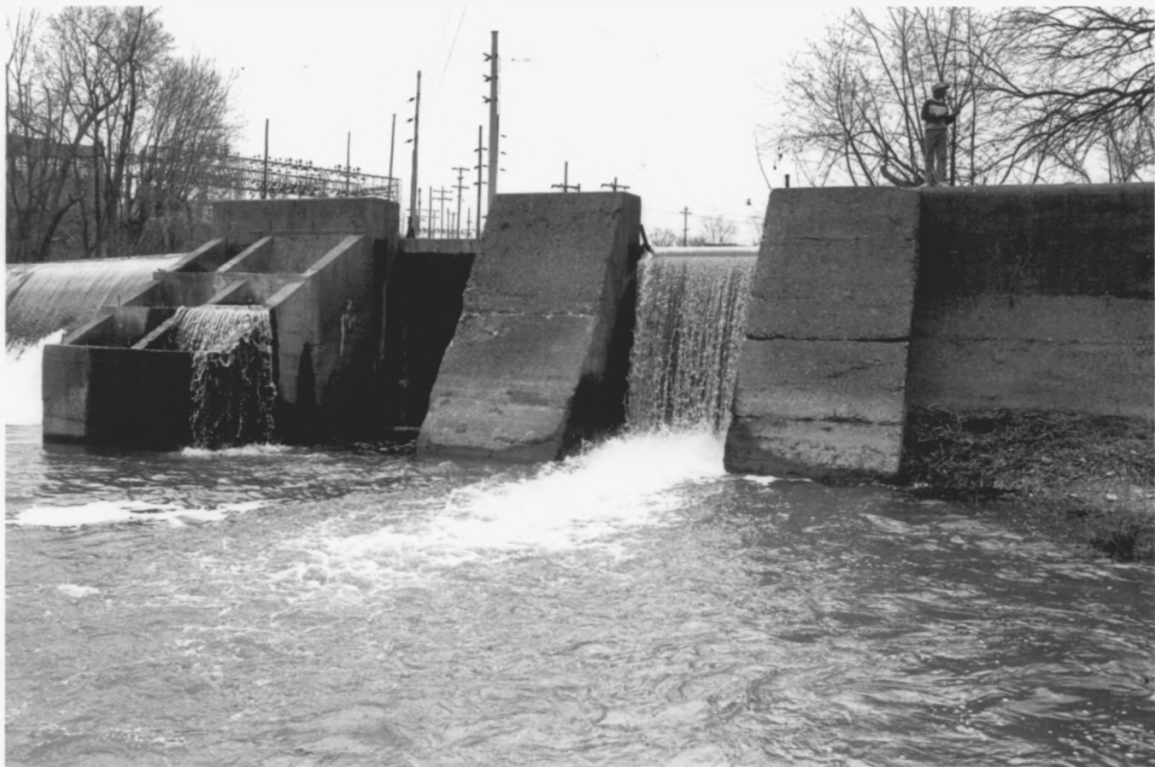
Shelbyville Hydroelectric Station Shelbyville, Bedford County, TN
