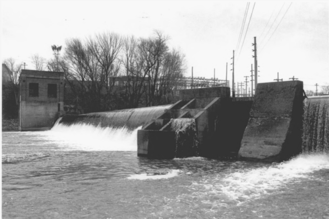
Shelbyville Hydroelectric Station Shelbyville, Bedford County, TN
