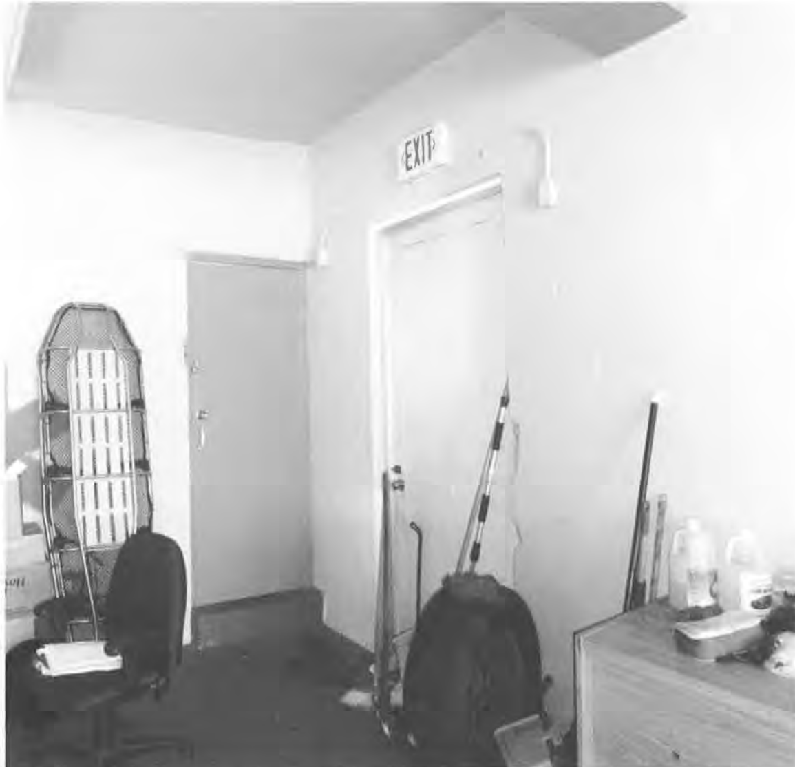
FIG. 7: Ceiba Fire Station south elevations, looking north. A side entrance door was added to provide a direct access to the side patio where a small gas tank storage closet had been added. Also a door was added to the first step of the stairwell to impede high-school students from going up to the second level. Photo: Guillermo Marrero, February 15, 2012. Source: Jorge Rigau Arquitectos, San Juan Puerto Rico.
