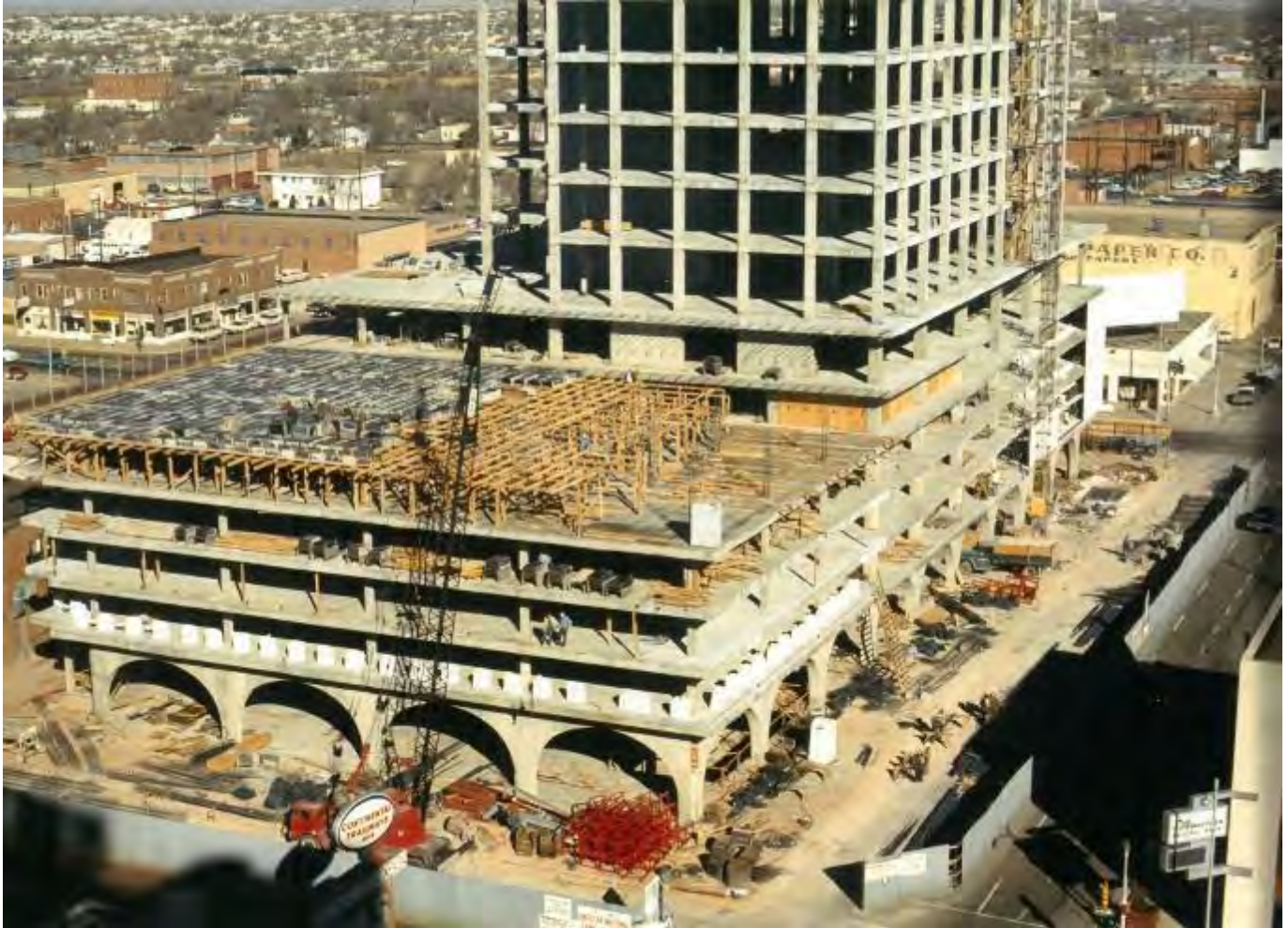
Figure 3: American National Bank Building and SPS Tower Under Construction, facing northwest c.1969 Source: Building Owner
