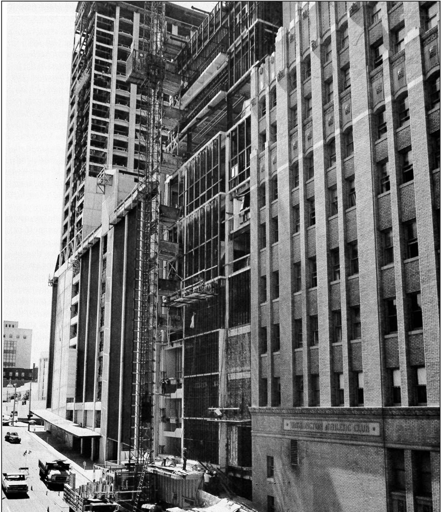
Ca. 1969. View looking south. Construction of eight additional stories on top of the 1955 four-story addition. The twelve-story addition was completed in 1970. The Hilton Hotel and parking garage is under construction at the end of the block in the foreground. Source: WAC
