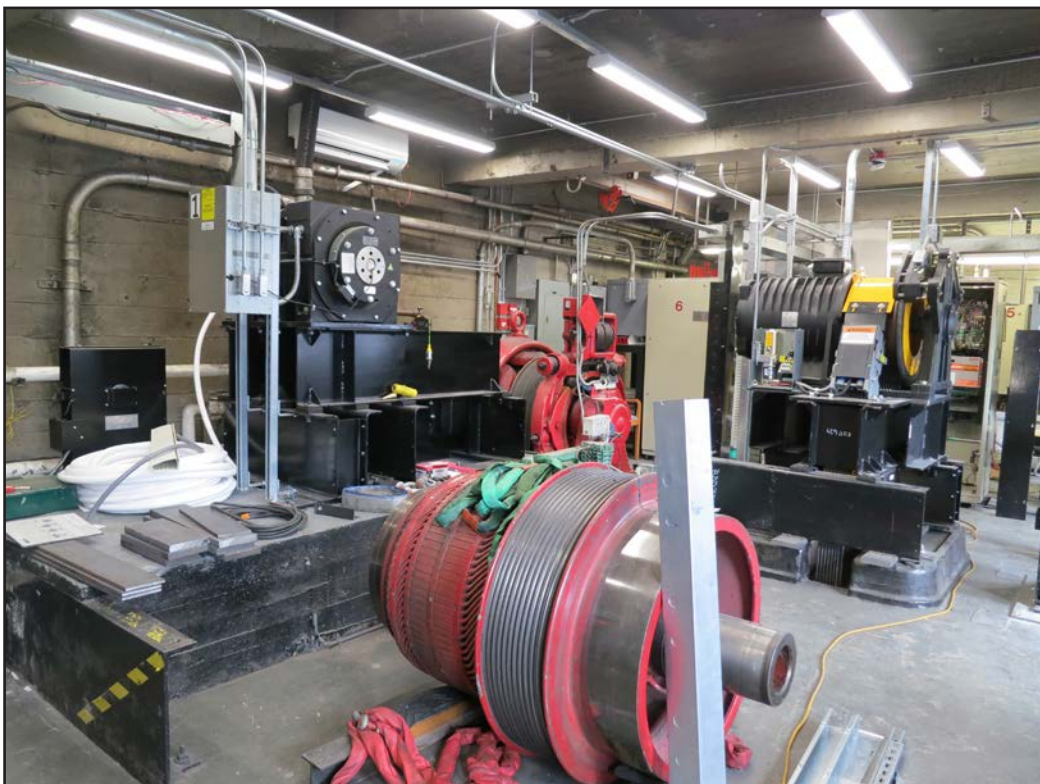
0056. Interior, elevator machine room - 23rd floor of original 1930 building.
