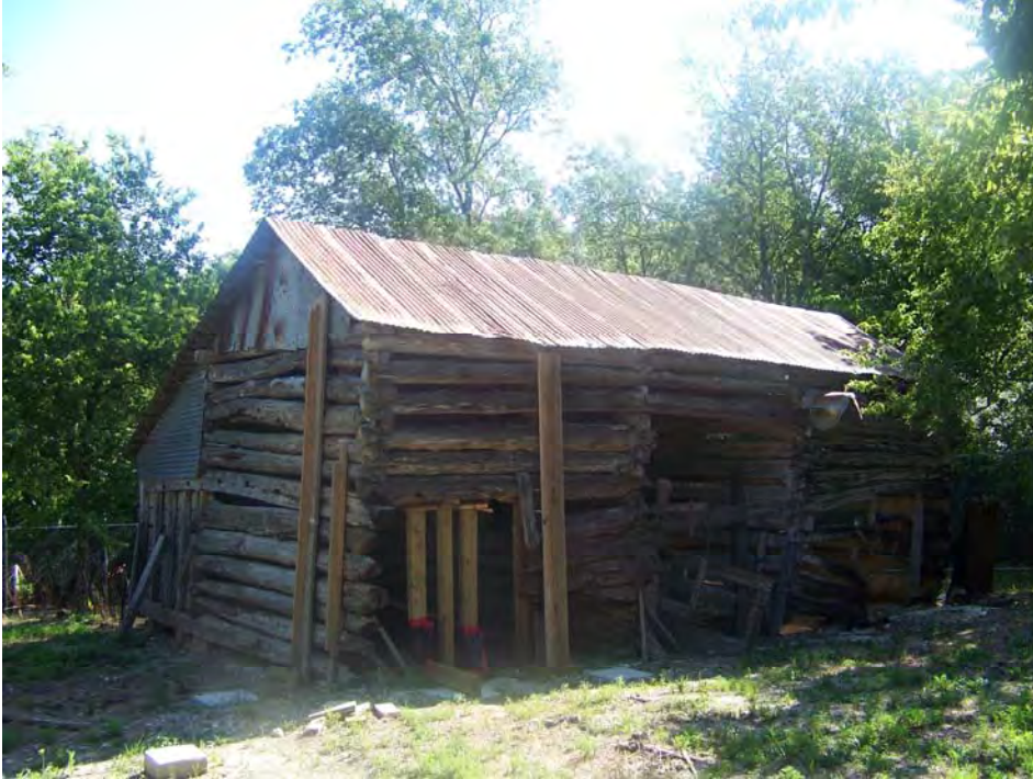
TX_Dallas County_ Everard Sharrock Jr. Farmstead_0004.tif Log Barn Southwest Oblique. Camera facing: Northeast
