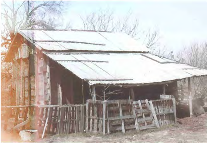
Figure 12 - Plank barn, March 1973, shows barn's appearance prior to collapse. Photo by Architect William Thomas Odum
