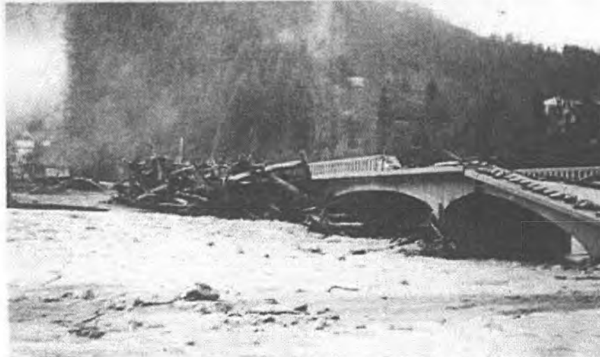
Remains of Highway Bridge
