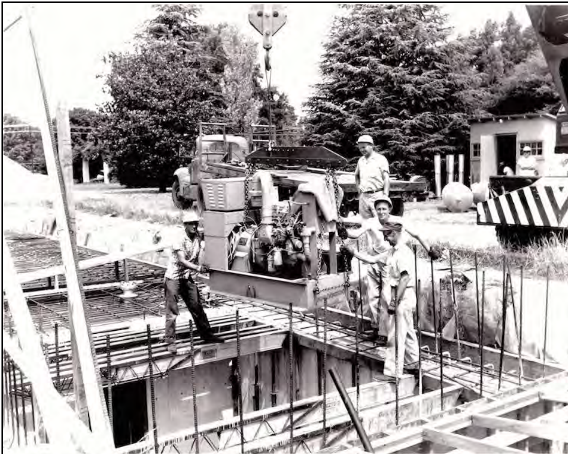
Figure 10: Construction of the Wooten Fallout Shelter and Installation of Generators, ca. 1962. Source: Vance Lauderdale, "Rare Photo: Wooten Bomb Shelter Being Constructed," Memphis Magazine , https://memphismagazine.com/ask-vance/rare-photo-wooten-bomb-shelter-being-constructed/ .
