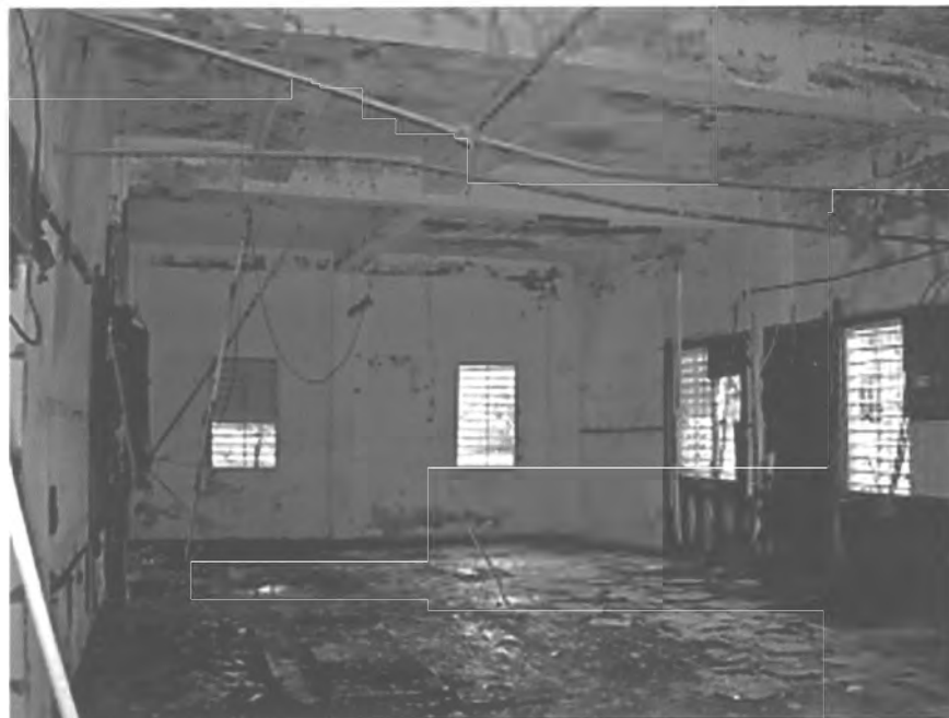
PHOTO #45. Valve and Mixing House, interior, Acueducto de San Juan Historic District.
