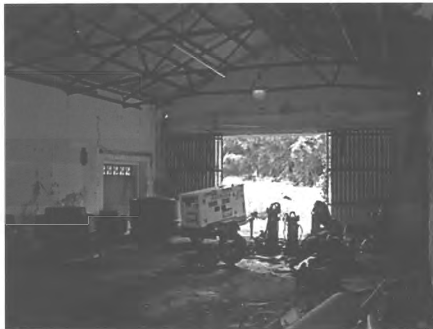
PHOTO #27. Pumping Station, coal store house, Acueducto de San Juan Historic District.
