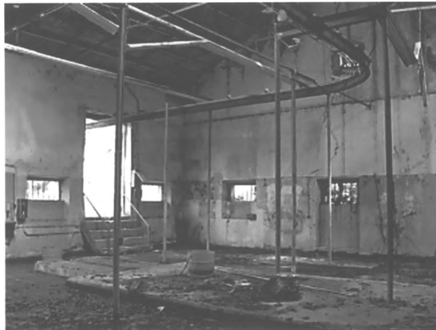
PHOTO #25. Pumping Station, interior, Acueducto de San Juan Historic District.
