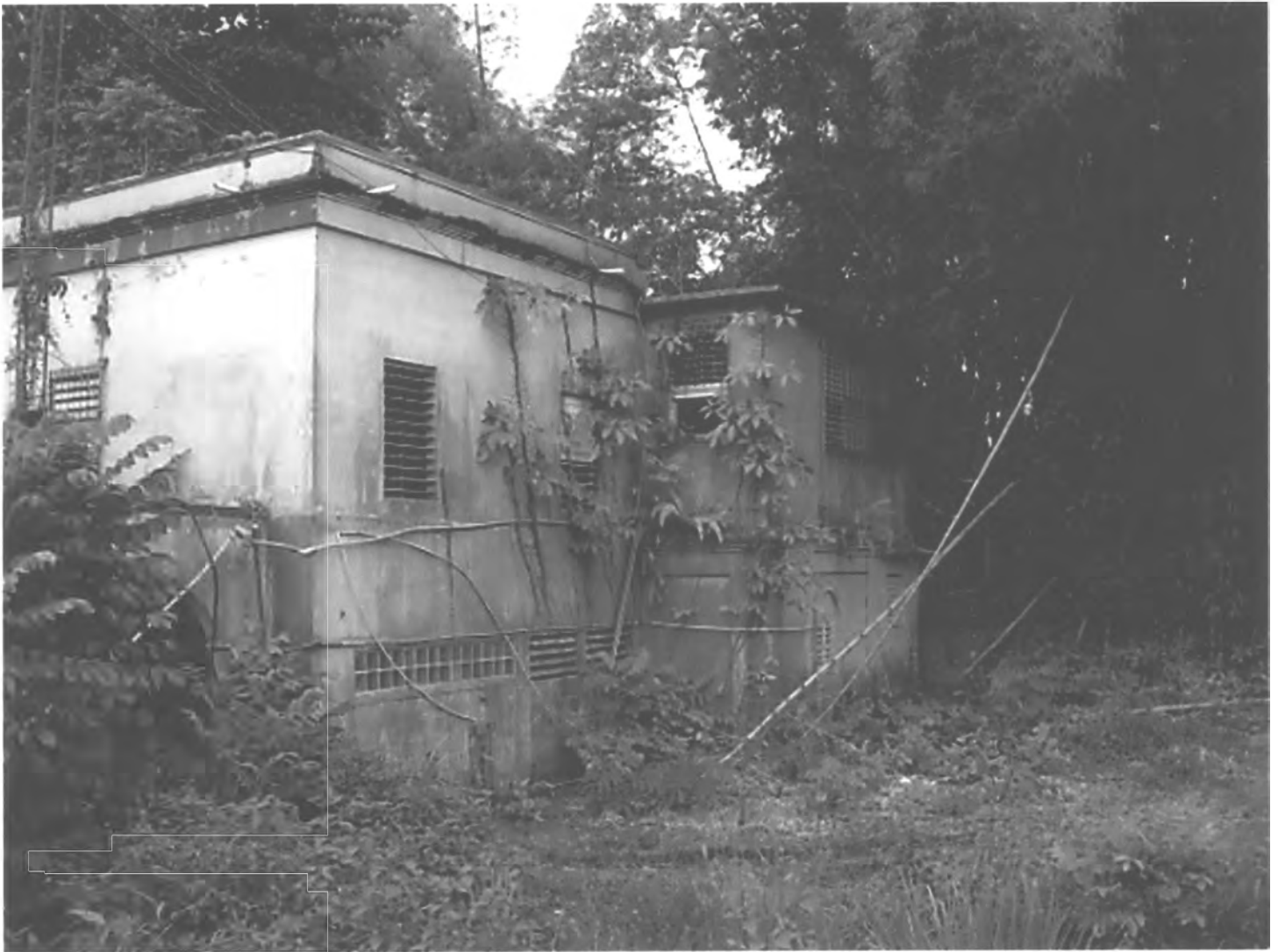
PHOTO #43. Valve and Mixing House, exterior, Acueducto de San Juan Historic District.
