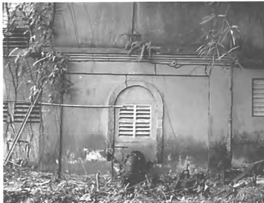
PHOTO #47. Valve and Mixing House, original building, Acueducto de San Juan Historic District.
