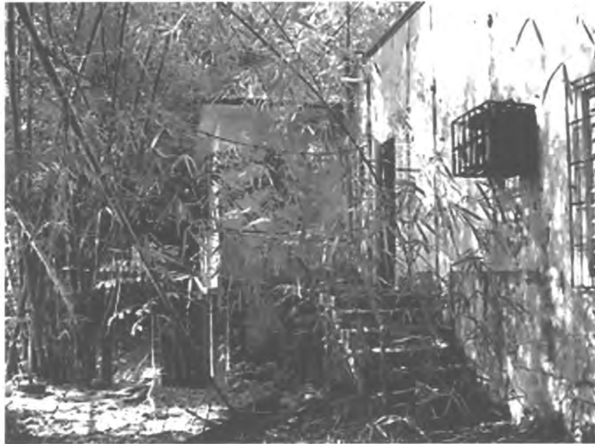
PHOTO #44. Valve and Mixing House, exterior, Acueducto de San Juan Historic District.
