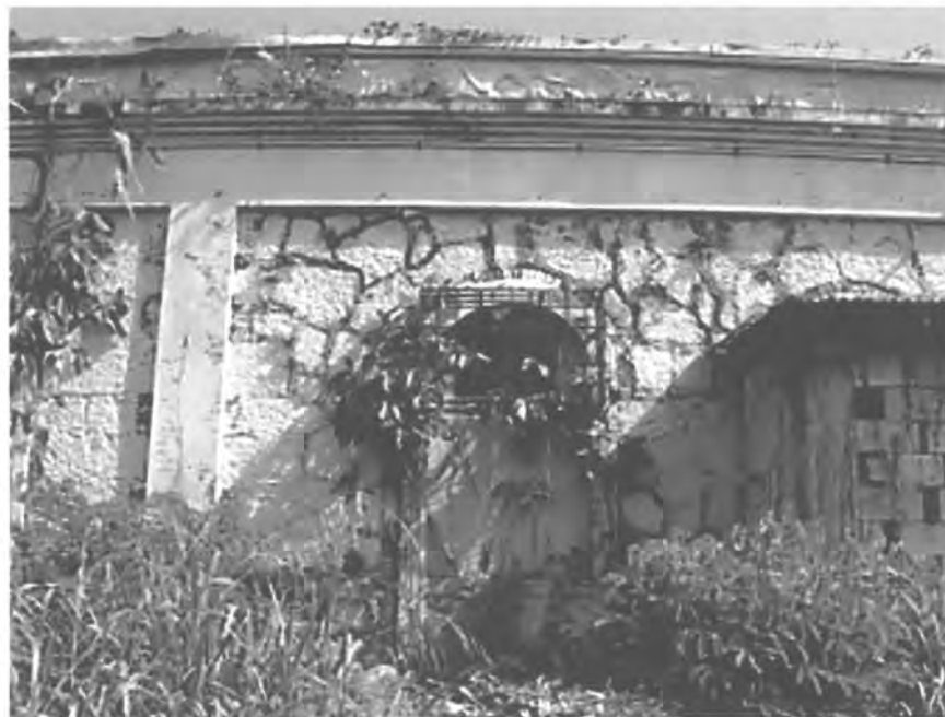
PHOTO #68. Engineers and Caretaker's Residence, wall detail, Acueducto de San Juan Historic District.
