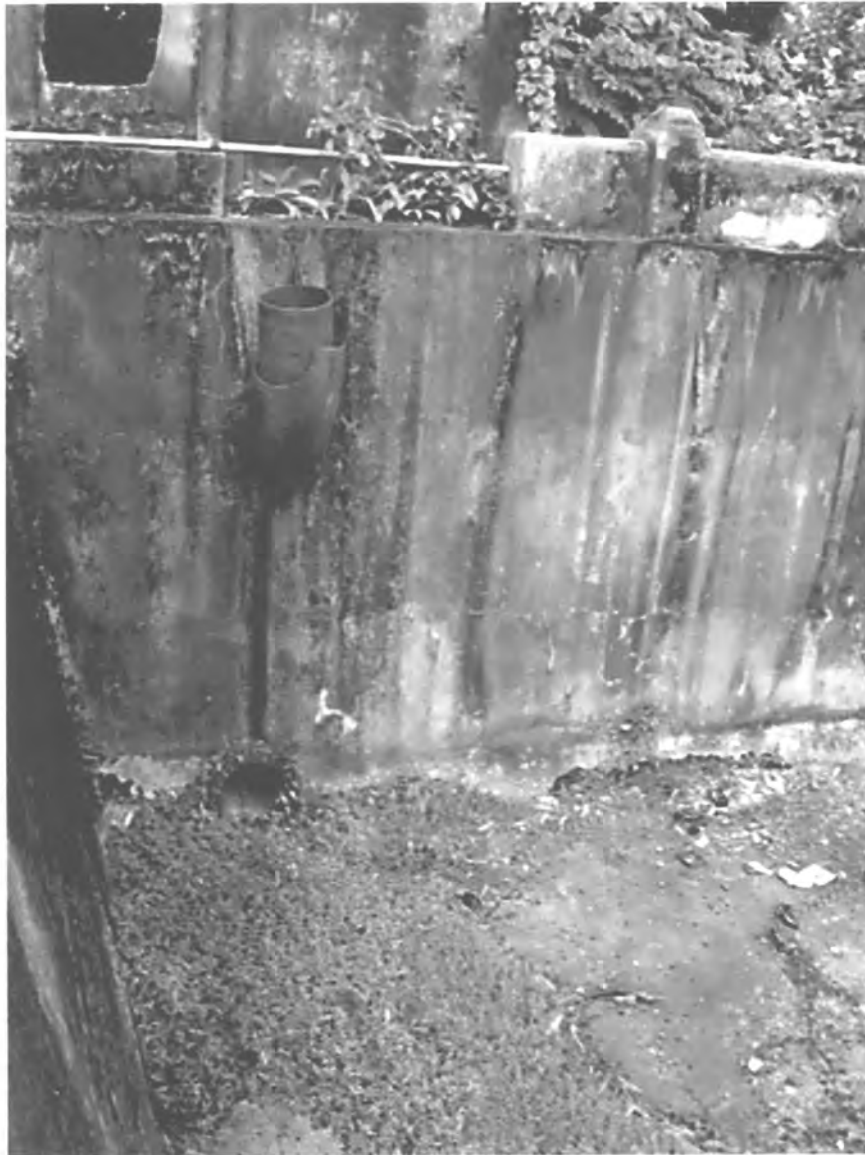
PHOTO #99. Water reservoir, intake and outtake pipes, Acueducto de San Juan Historic District.
