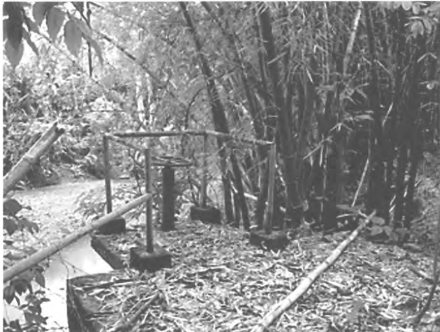
PHOTO #49. Valve and Mixing House, exterior intake valve, Acueducto de San Juan Historic District.
