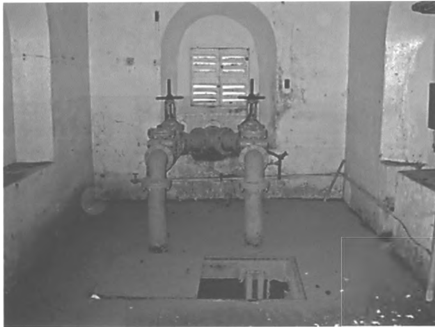
PHOTO #46. Valve and Mixing House, Valves, Acueducto de San Juan Historic District.
