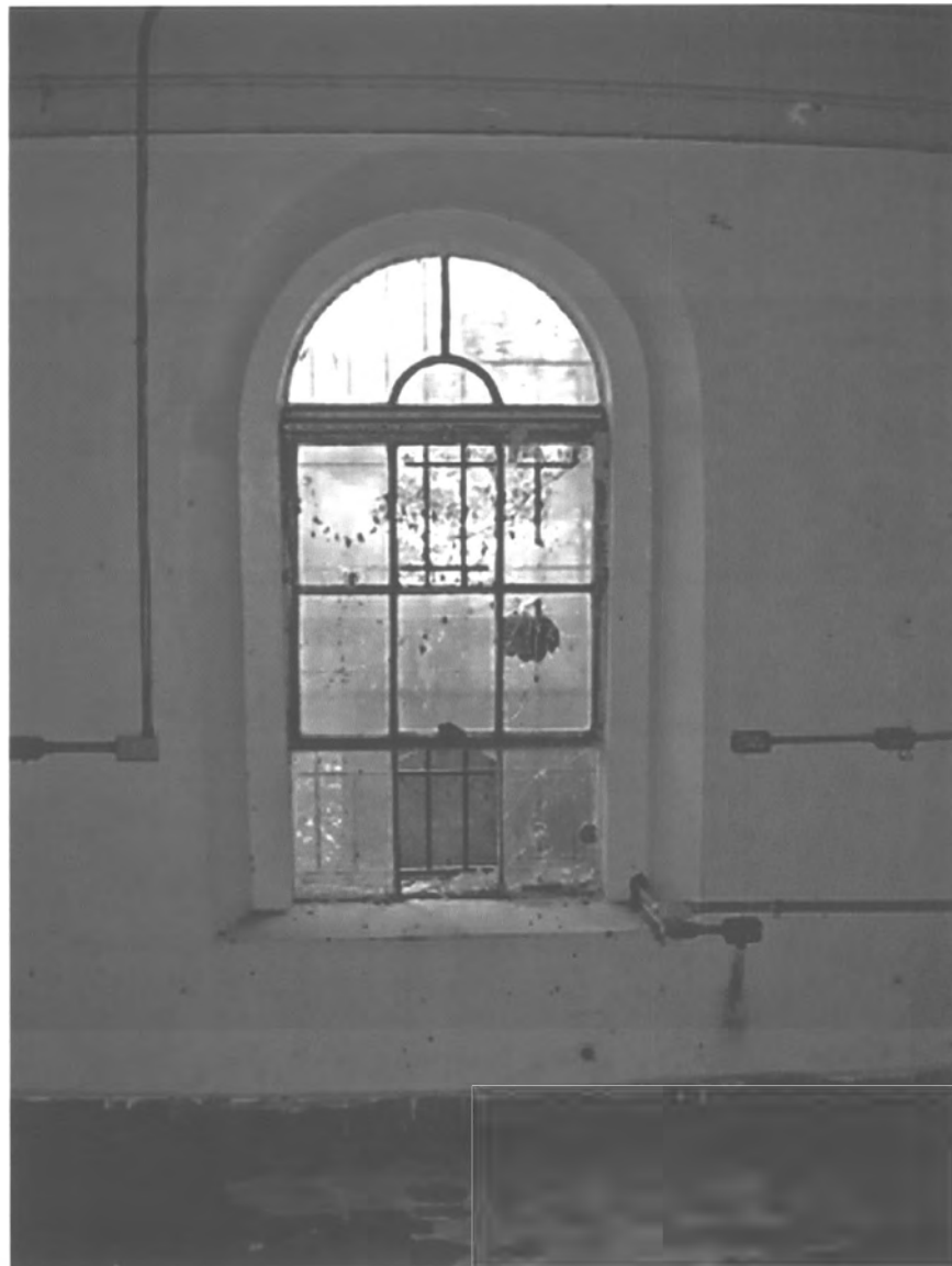
PHOTO #71. Engineers and Caretaker's Residence, window, Acueducto de San Juan Historic District.
