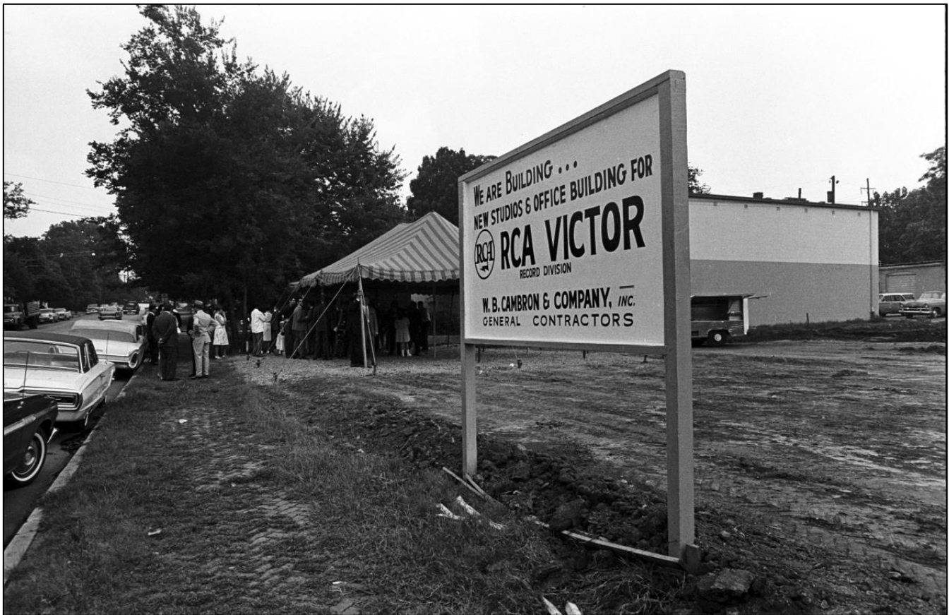
This photo from 1964 shows the construction site on the day of the groundbreaking ceremony. Photo courtesy of Grand Ole Opry Archives.
