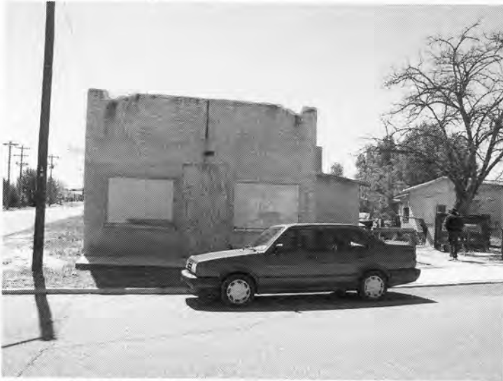
Photo 17. Former Deliciosa Café, now vacant, built around 1936. Owners Diego and Angelita Guitierrez ran a restaurant and package liquor store from the premises. Built of stuccoed adobe, this corner store has large storefront windows, a central entry and sculpted parapets.
