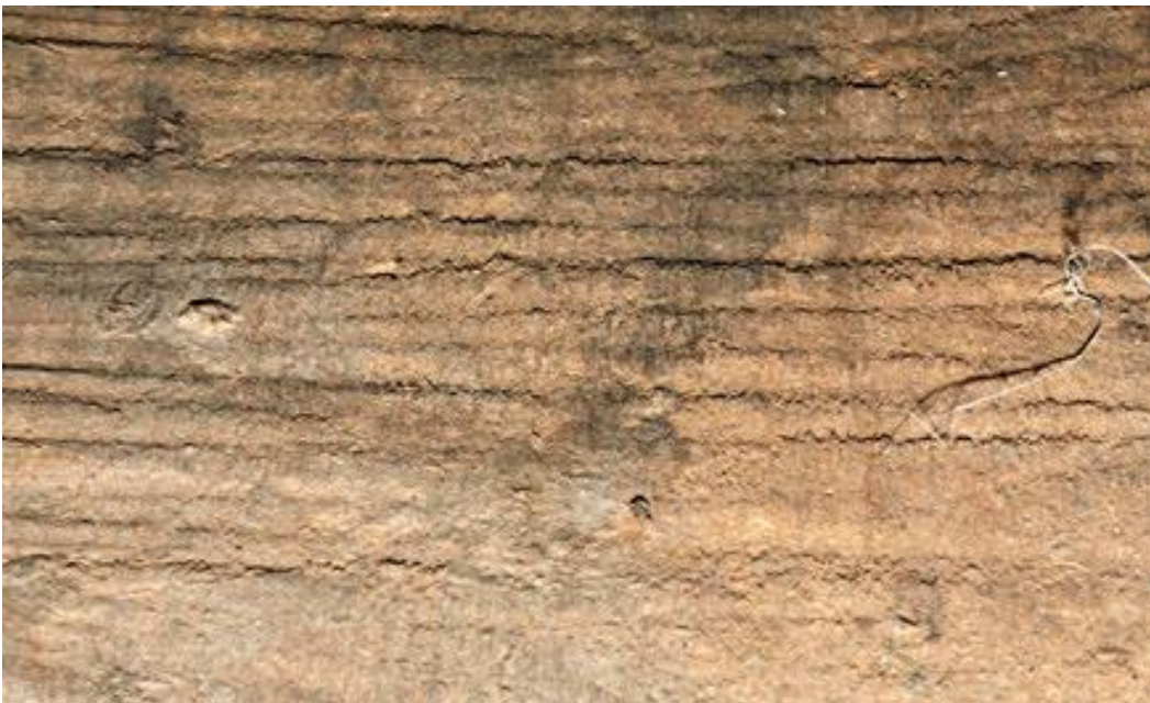
Photo 8: Typical pit saw marks found in early sections of Sellers Hall (University of Pennsylvania, 2010).
