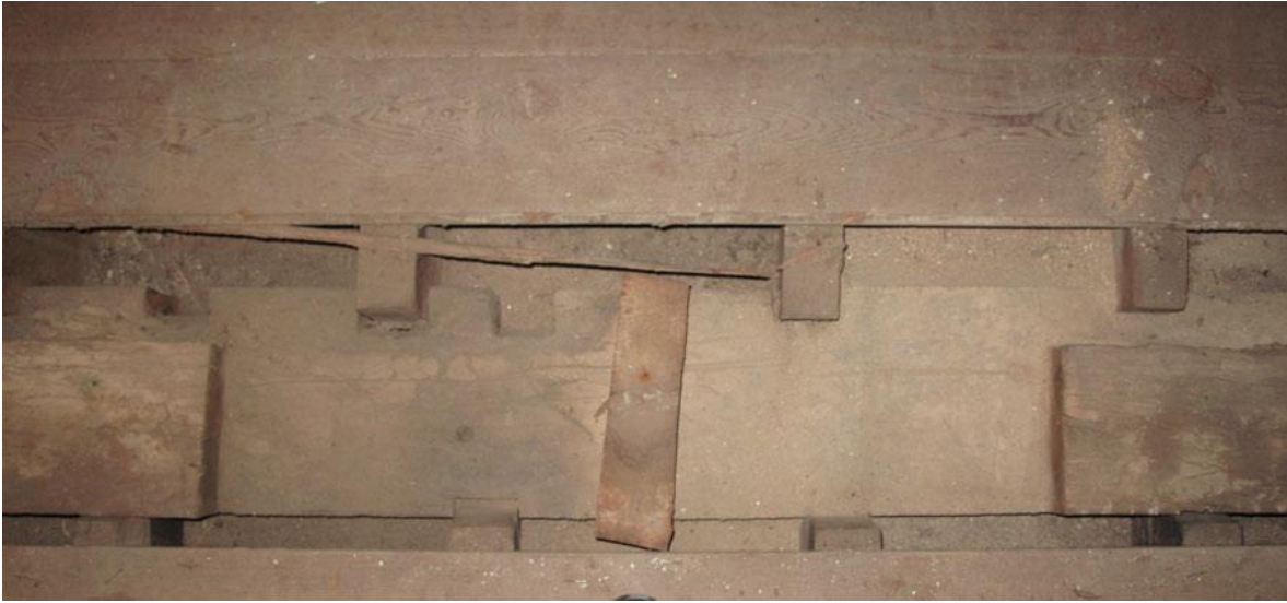
Photo 15: Summer beam with notch cut into it locating the original placement of the hearth (University of Pennsylvania, 2011).
