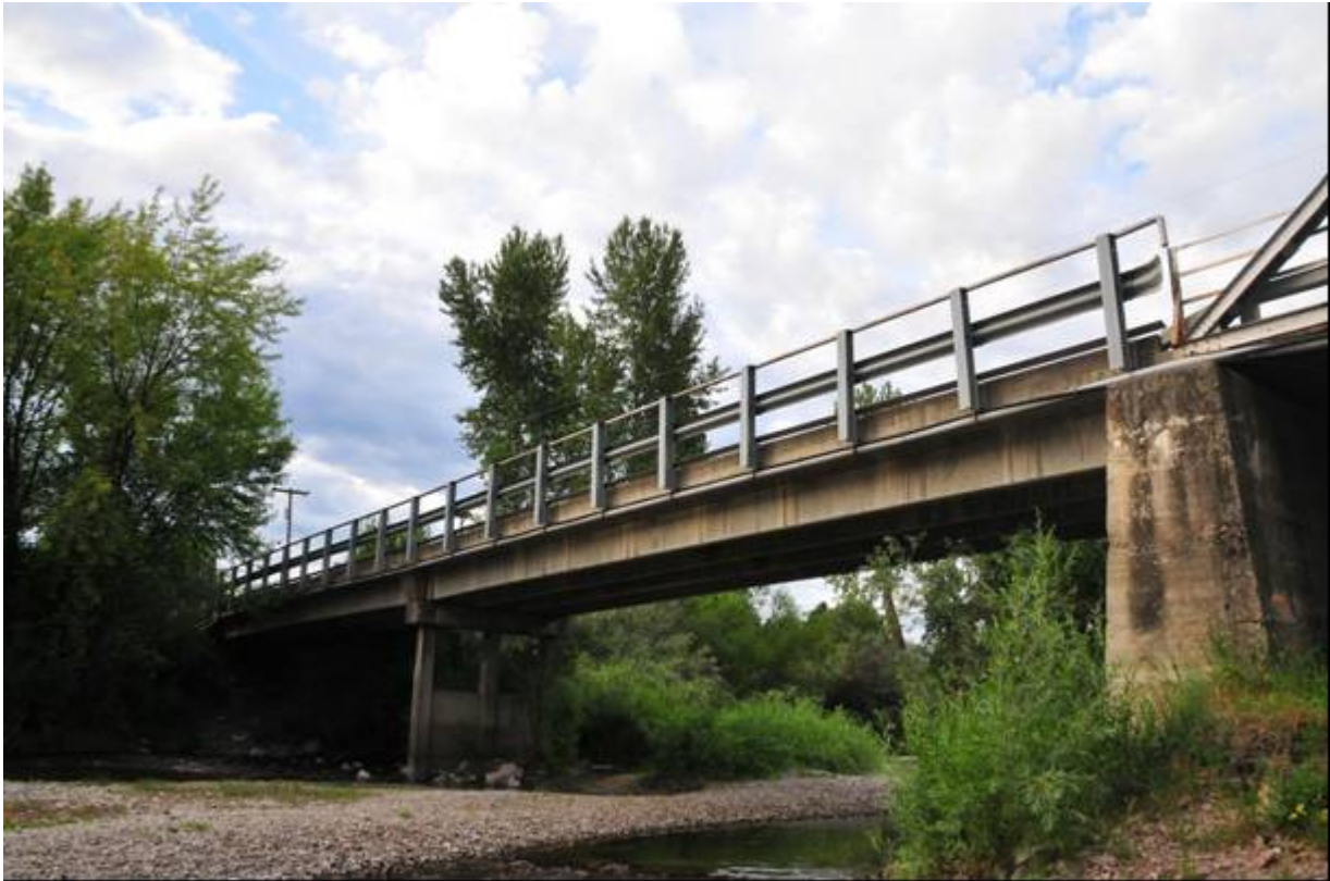
Photo MT_MissoulaCounty_MaclayBridge_0004 (4 of 9) Maclay Bridge: view to the south showing the two prestressed concrete T-beam approach spans: columnar type concrete pier mid span and solid concrete pier to the right where the span joins the southeast end of the Warren pony truss.
