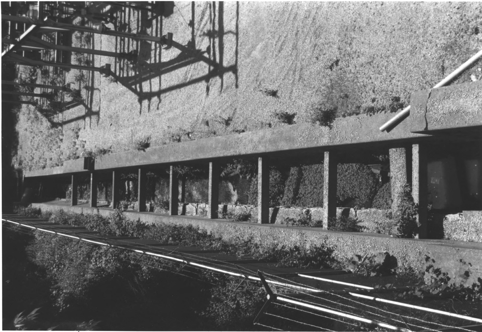
LOG SLUICE ST. ANTHONY FALLS HISTORIC DISTRICT MINNEAPOLIS, HENNEPIN CO., MN PHOTO: 010264-10
