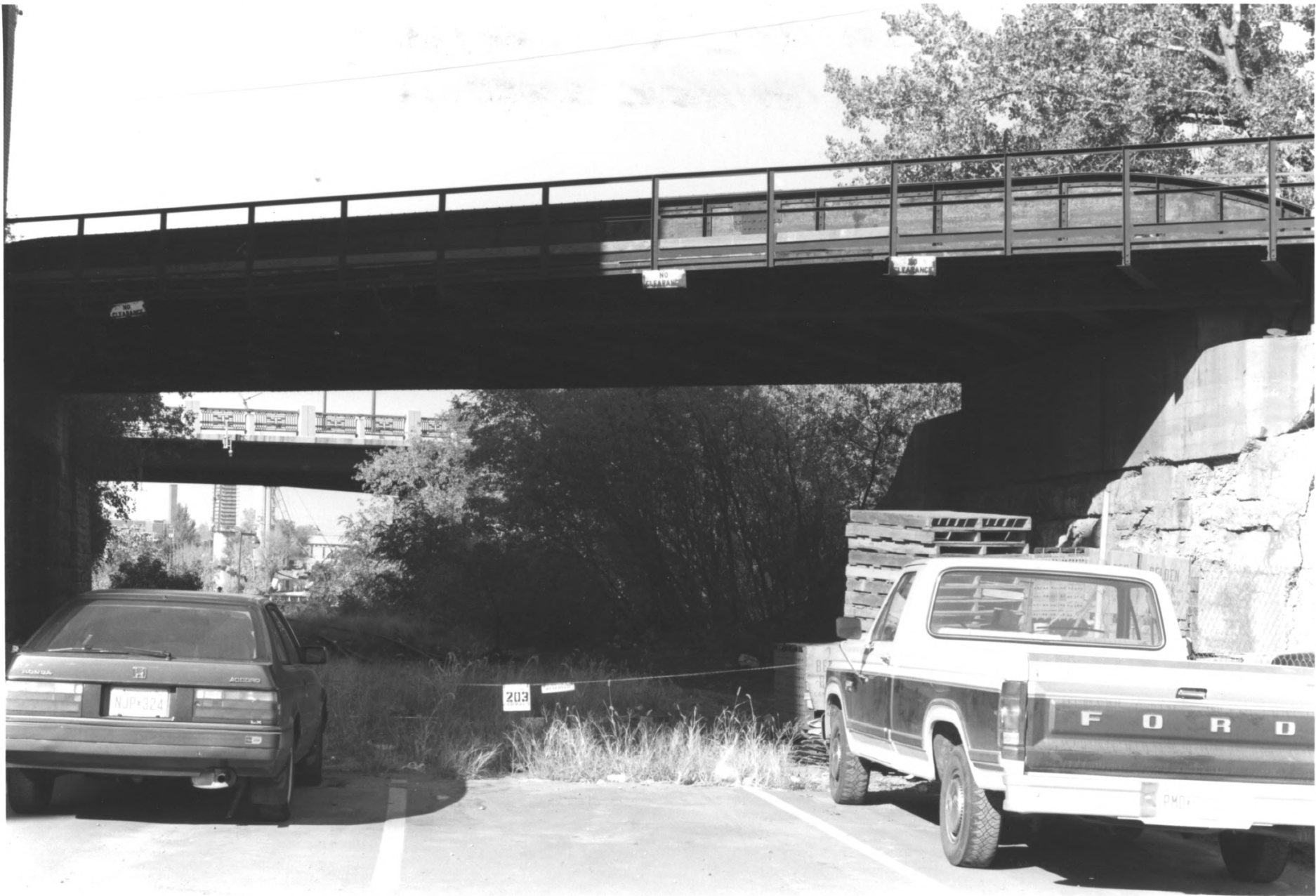
RAILROAD BRIDGE NO. L 8900 ST. ANTHONY FALLS HISTORIC DISTRICT MINNEAPOLIS, HENNINGEN CO., MN PHOTO: 010055-6
