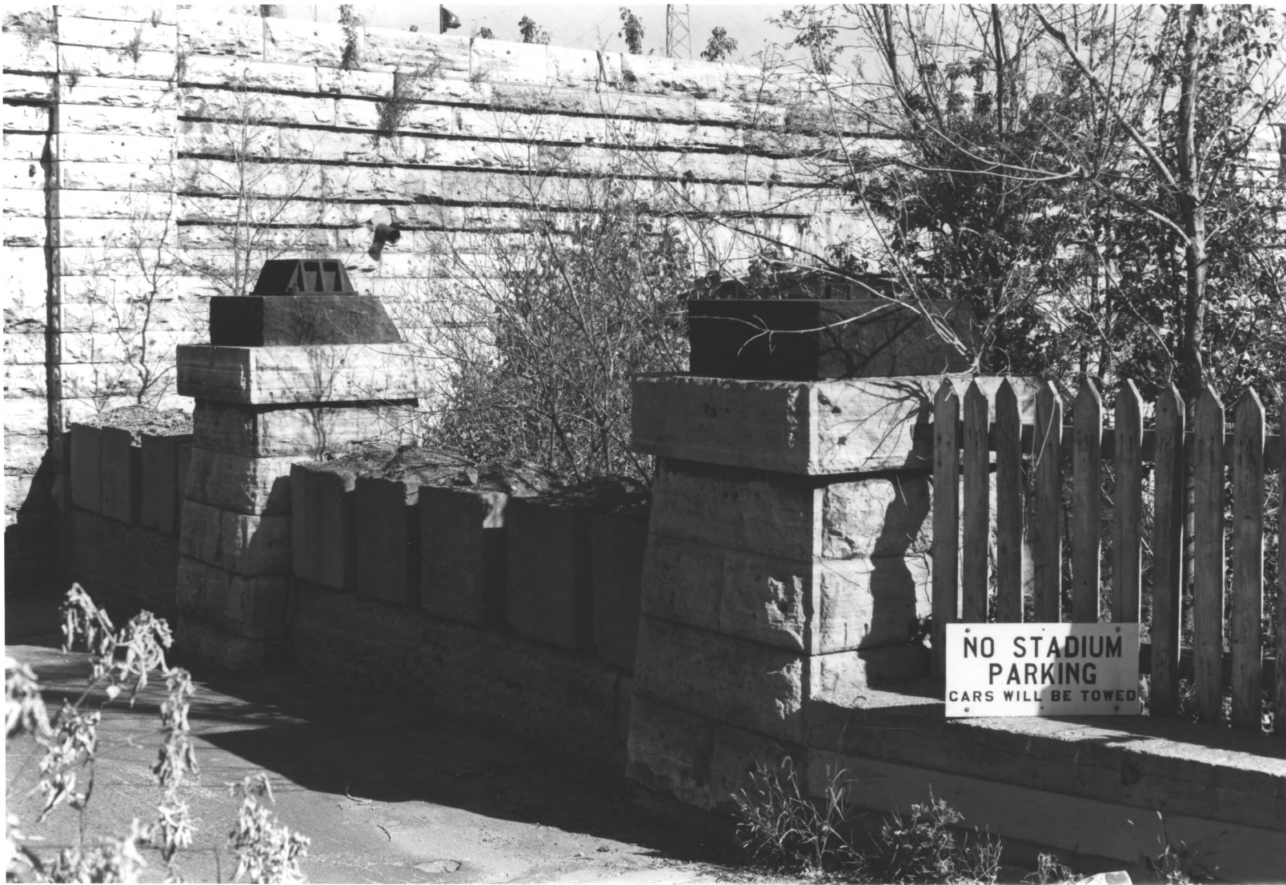
MINNEAPOLIS EASTERN RAILROAD TRESTLE PIERS ST. ANTHONY FALLS HISTORIC DISTRICT MINNEAPOLIS, HENNEPIN CO., MN PHOTO: ©10056-7
