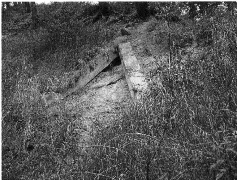
Photo# 0016 Concrete buttressing on the east slope (top); near carriage path. View to the east.
