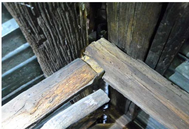
The rafter peaks were joined with open mortise and tenon joints, a very common method for joining rafters together except there was never any pegs. The lack of pegs here is very usual.
