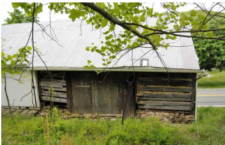
The rear elevation from the hillside above the shop, showing the wagon access-area into the upper level. The wagon doors are currently covered by plywood.
