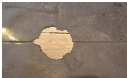
Looking down from the loft through the stove pipe opening. Two of the three metal spacers remained nailed to the flooring. Charred edges of the flooring indicate hot conditions existing, and flooring was overheated.
