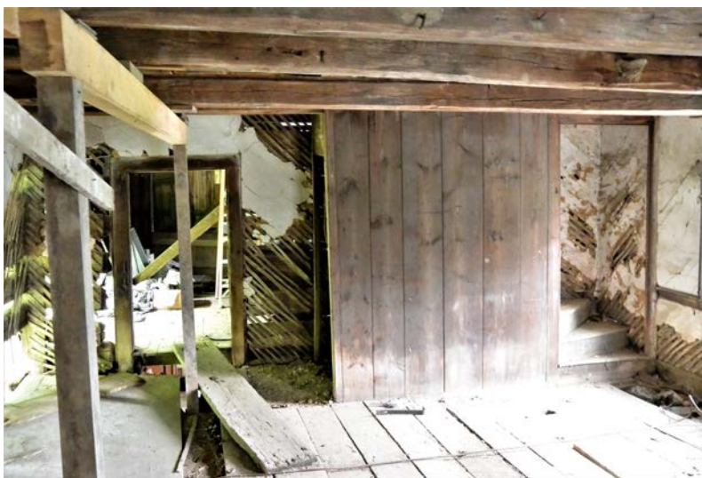
Staircase connecting the second floor interior to the loft, with former exterior Dutch door opening to the left of the staircase.
