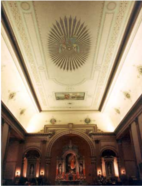
FIGURE 26. NAVE CEILING BEFORE HANGING OF SAFETY NETTING IN 1989 (PHOTO 2005, COURTESY KATHERINE PETRIN).
