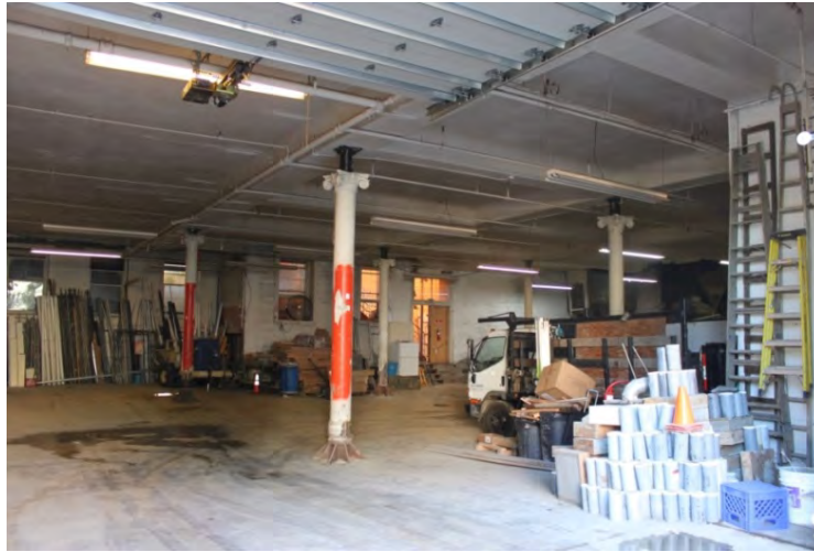
FIGURE 12. CHURCH: BASEMENT SHOWING GUTTED CONDITION, 2015.
