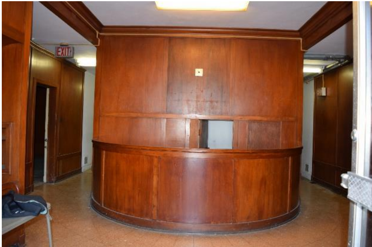
Photo 17 – Interior showing original finishes in Building #13, view east towards the first floor lobby, February 2017.
