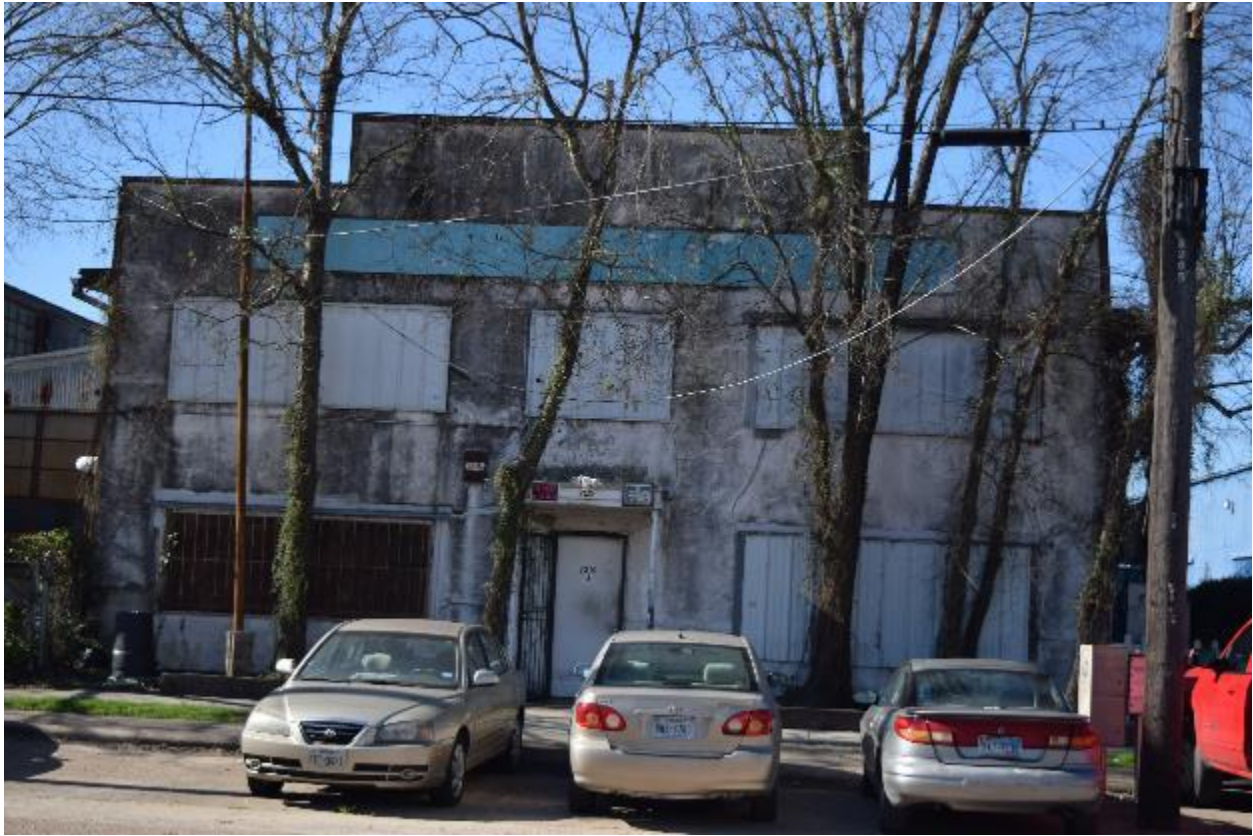
Photo 4 – North (front) elevation of Building #2, #3, and #4. Window, door, and signage alterations visible, camera facing south, February 2017.
