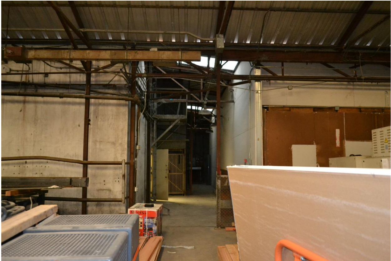
Photo 19 – Covered space between Building #13 (left) and Building #14 (right), taken from inside Building #15, view west, October 2017.
