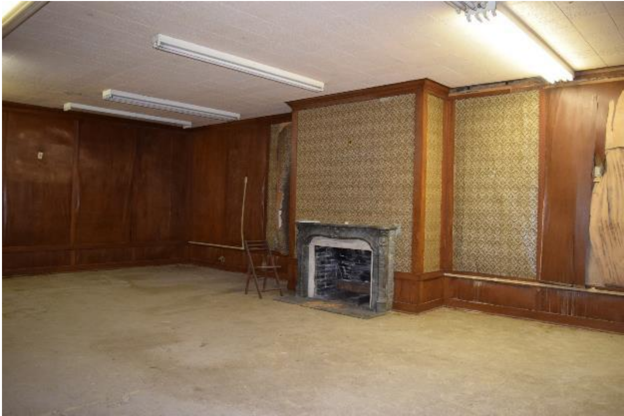
Photo 18 – Second floor conference room in Building #13 showing original ceiling, fireplace, and wood paneling, view south, February 2017.
