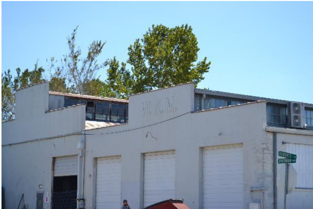
Photo 11 – Detail of remaining W-K-M signage on the north elevation of Building #10, view southeast, September 2017
