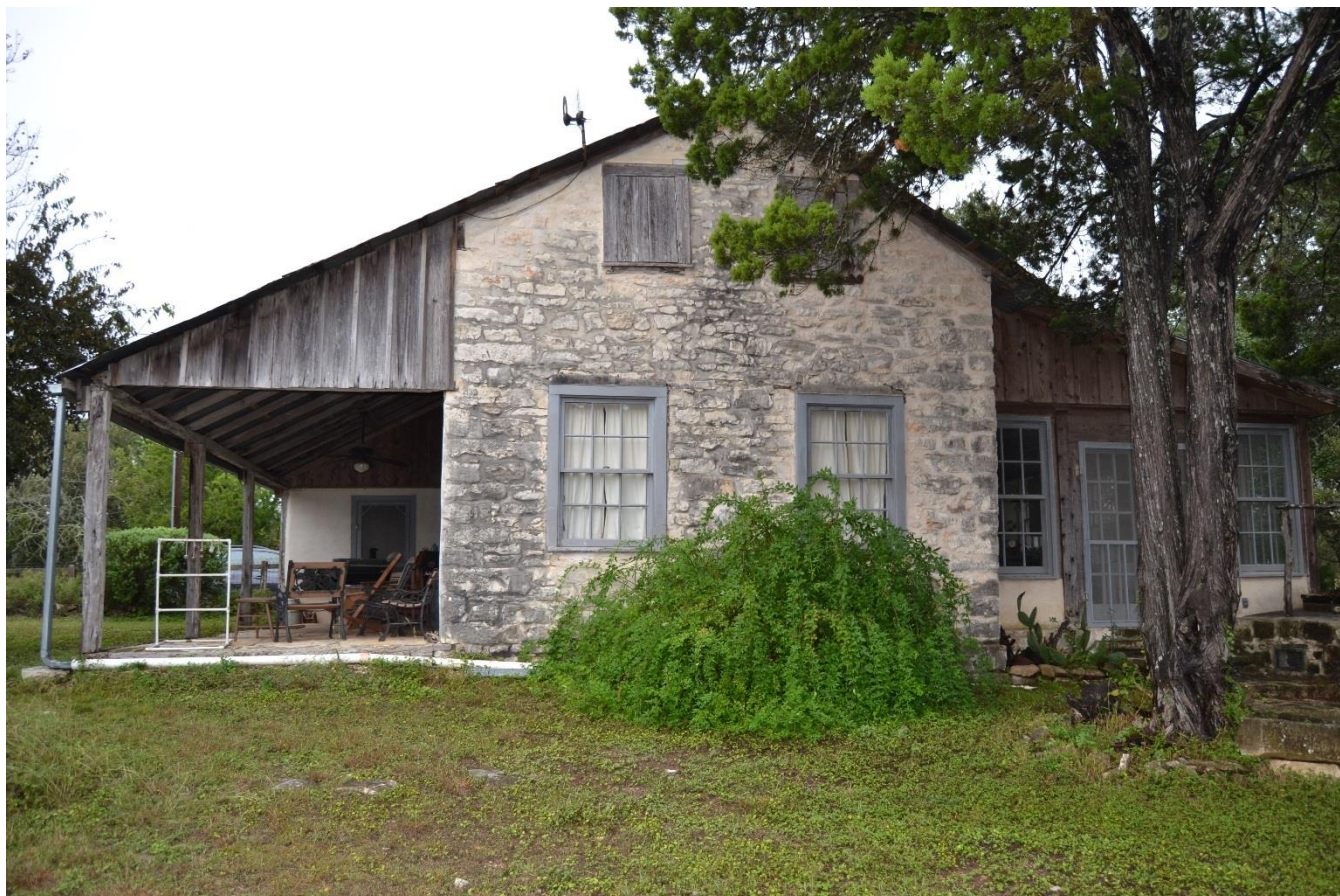
Photo No. 9. Side east façade of house (RIDN 81039 a) showing rubble stone, view facing west.
