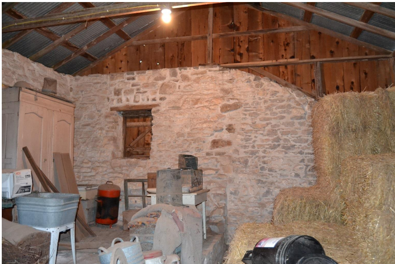
Photo No. 26. Partial stone wall in middle of barn (RIDN 81039 b), view facing southwest.
