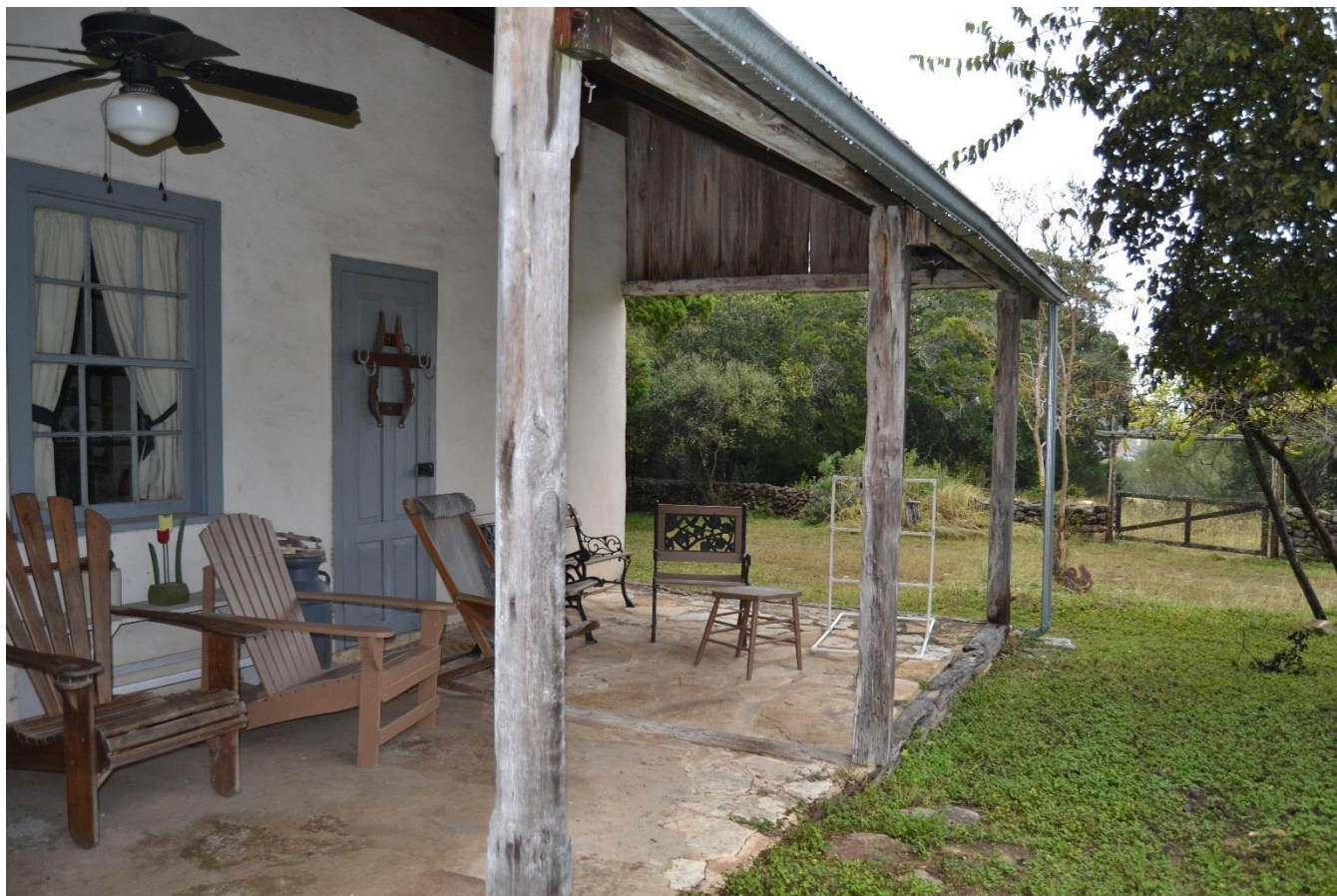
Photo No. 11. View showing chamfered porch columns on house (RIDN 81039 a), view facing east.
