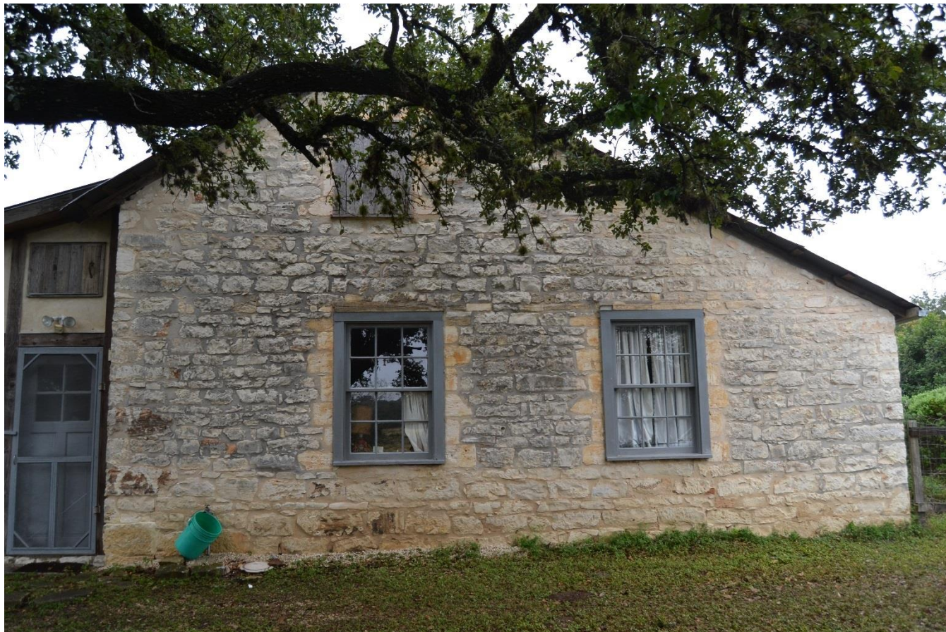
Photo No. 10. Side west façade of house (RIDN 81039 a) show cut limestone, view facing east.
