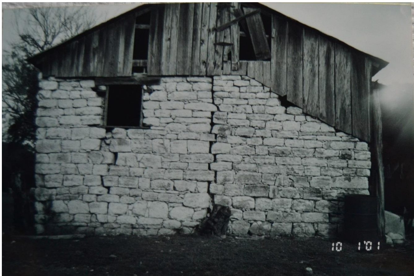
Figure 6. Photograph from 2001 showing the side west façade. Notice the north and side sides separating from one another. Source: Alton Rahe.
