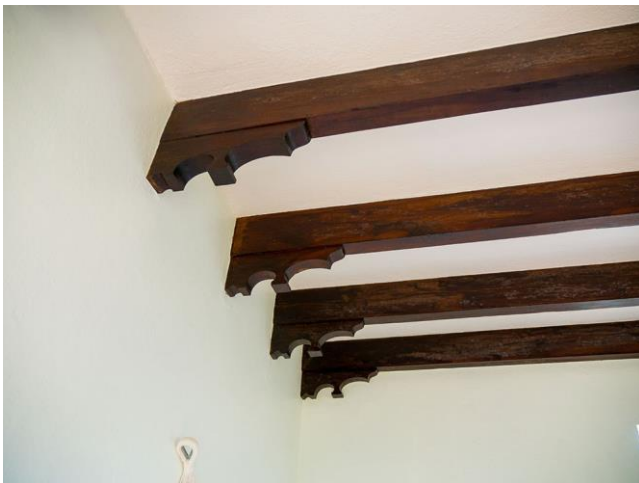
Figure 9: Detail of exposed wood beams in the fourth floor of the tower (looking west), 2017.
