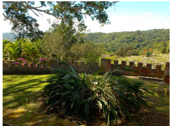
Figure 62: Detail of the merlons that replaced the original wrought iron rail (looking southeast), 2017.
