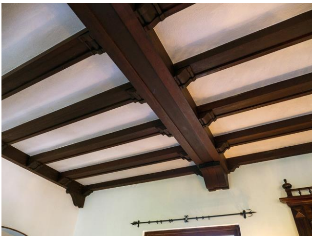
Figure 25: Detail of the alfarje (paneled ceiling) in the living room (looking east), 2017.
