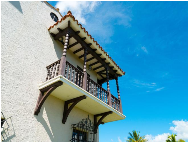
Figure 7: Detail of the roofed corner balcony at the main façade (looking northwest), 2017.
