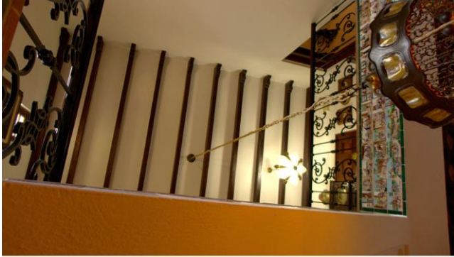
Figure 47: View of the exposed wood structure on the ceiling of the main staircase (looking up), 2017.
