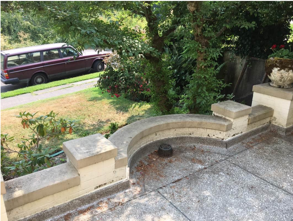
Photo #24 of 25 (WA_King County_Hannah Lewis House_0024) Patio, primary elevation, camera facing southeast
