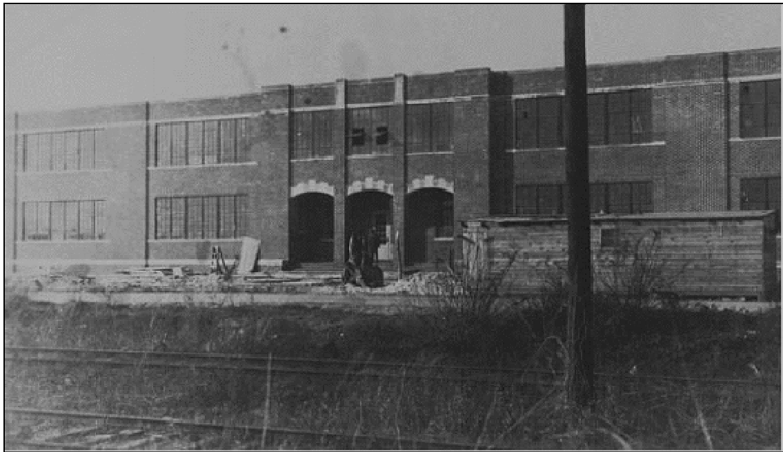
11. Construction Photograph of the 1926 Oceana High School (Source: Library of Virginia, School Buildings Service of the Virginia Department of Education)
