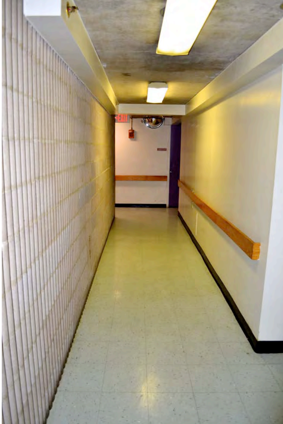
Detail of typical upper-floor corridor, showing floor, wall, and ceiling details. Camera facing southeast. Photograph 17 of 19.
