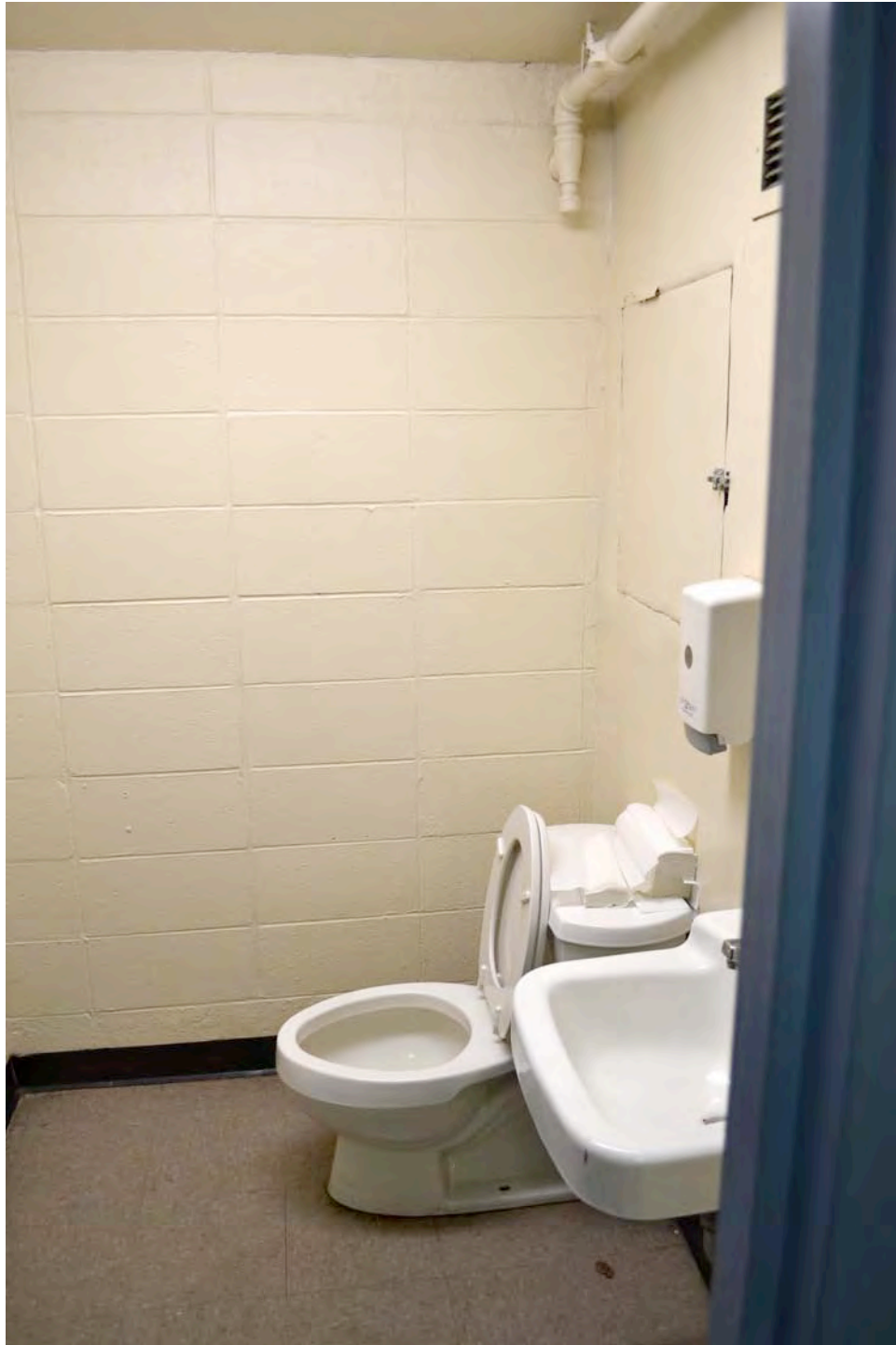
Detail of first-floor restroom, showing floor, wall, and fixture details. Camera facing northeast. Photograph 10 of 19.
