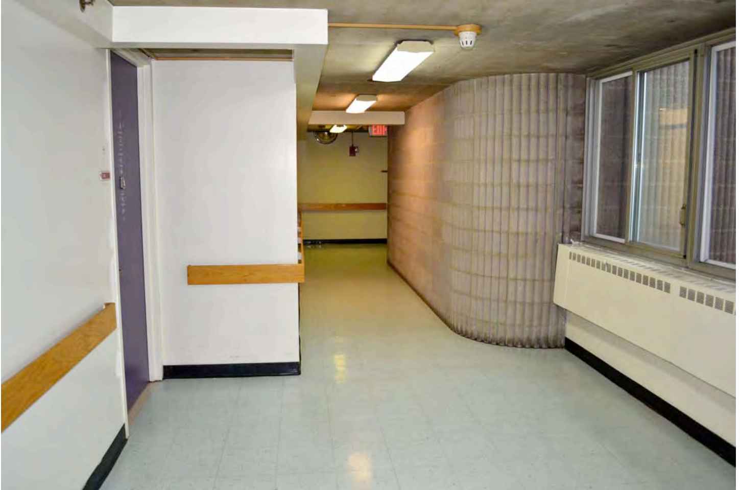
Detail of typical upper-floor corridor, showing floor, wall, and ceiling details. Camera facing northwest. Photograph 16 of 19.
