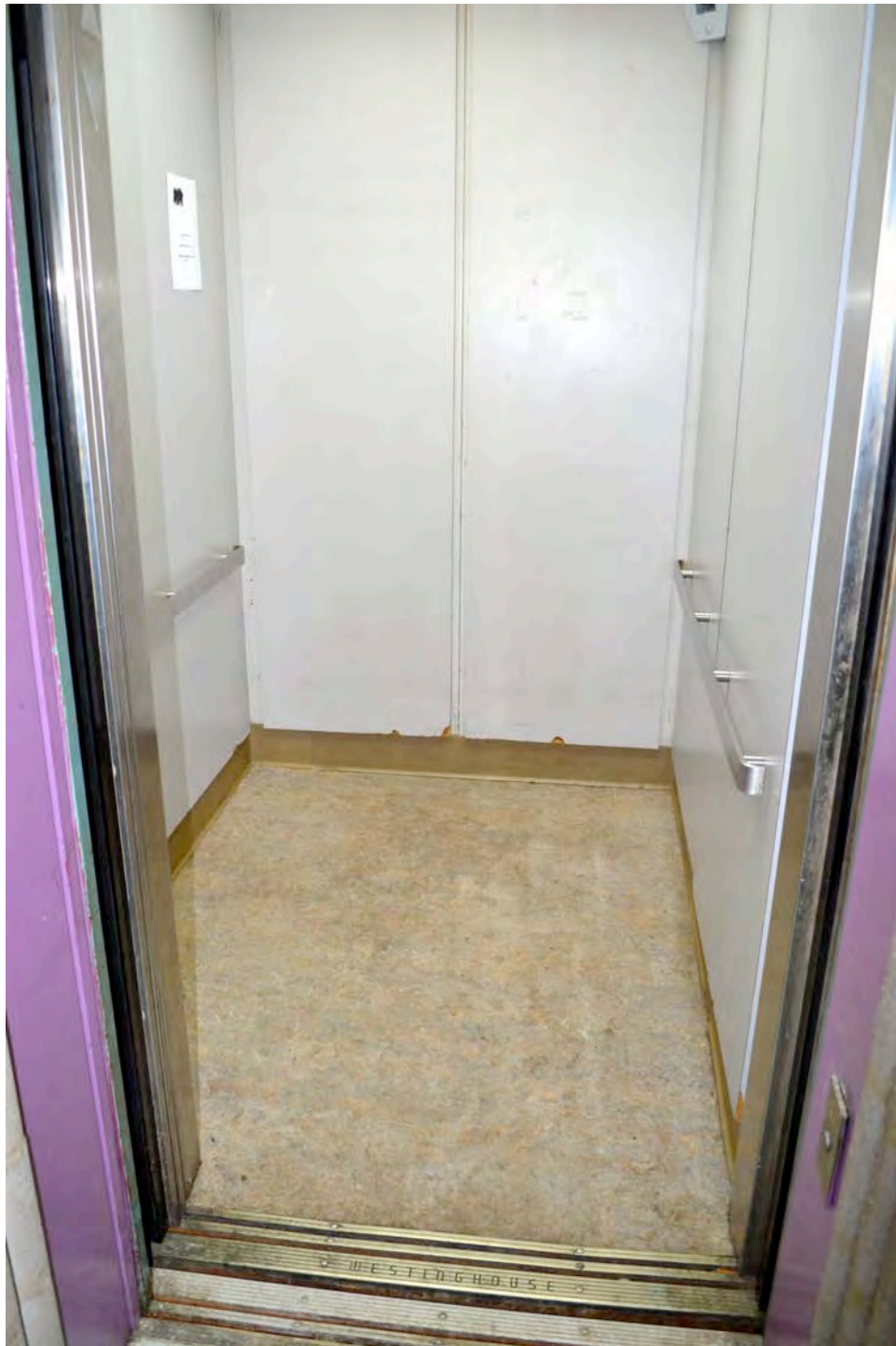
Detail of typical upper-floor elevator car, showing floor and wall details. Camera facing southeast. Photograph 14 of 19.
