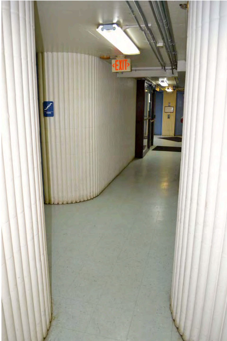
Detail of first-floor entry and corridor, showing floor, wall, and ceiling details. Camera facing east. Photograph 7 of 19.
