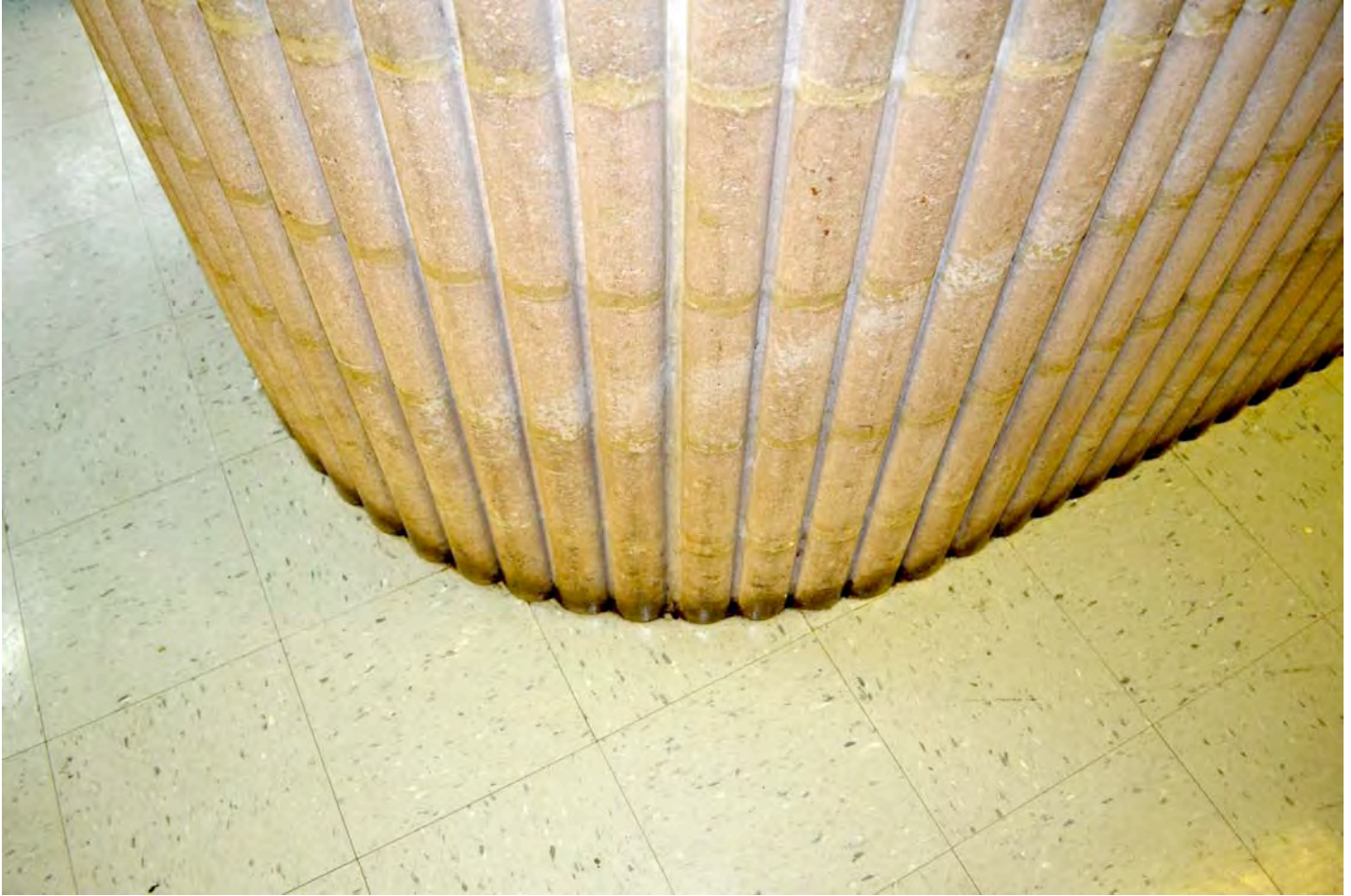
Detail of typical upper-floor corridor wall, showing ribbed concrete block details. Camera facing northeast. Photograph 19 of 19.
