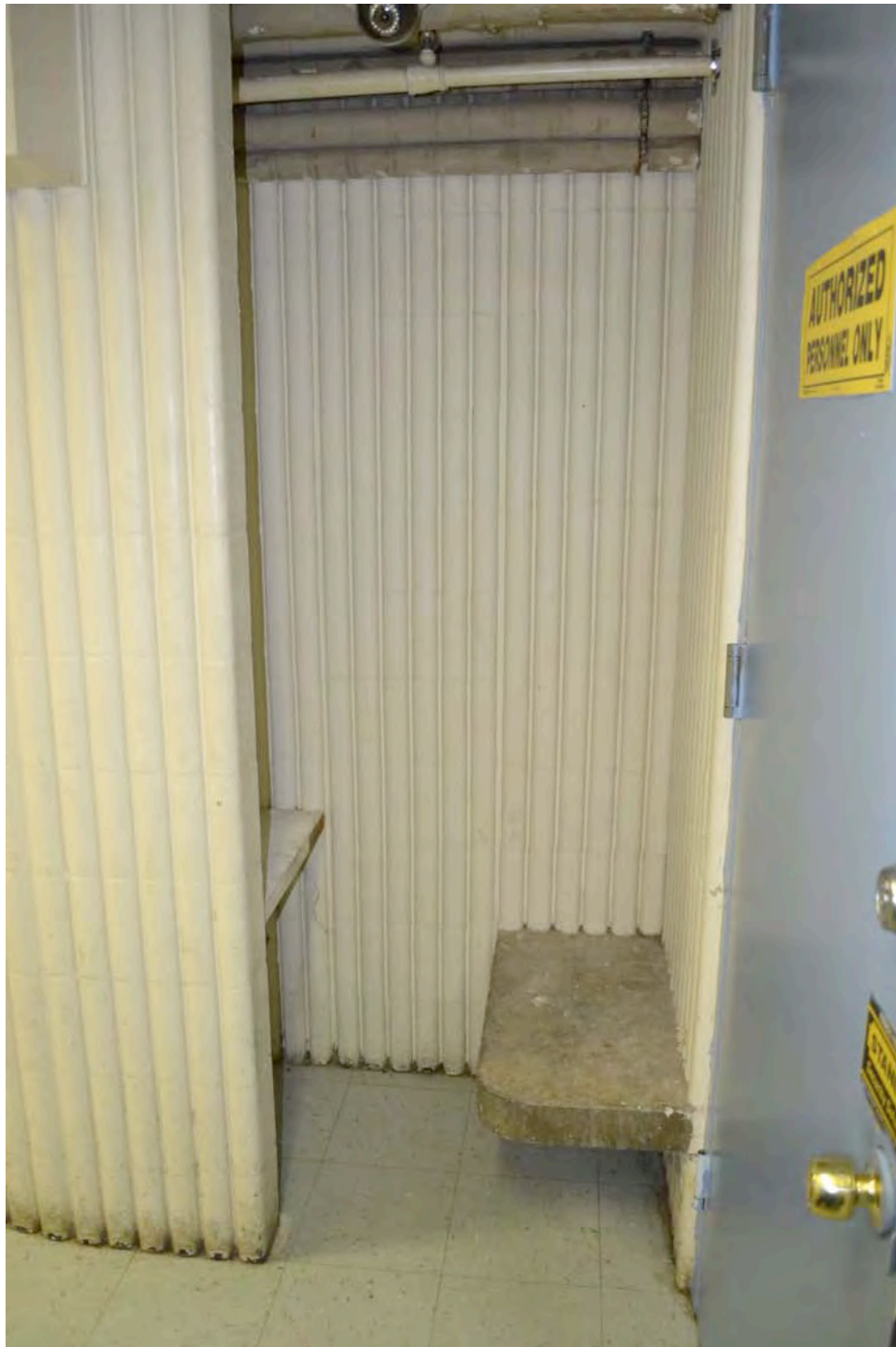
Detail of first-floor pay phone nook, showing floor, bench, and wall details. Camera facing southeast. Photograph 9 of 19.
