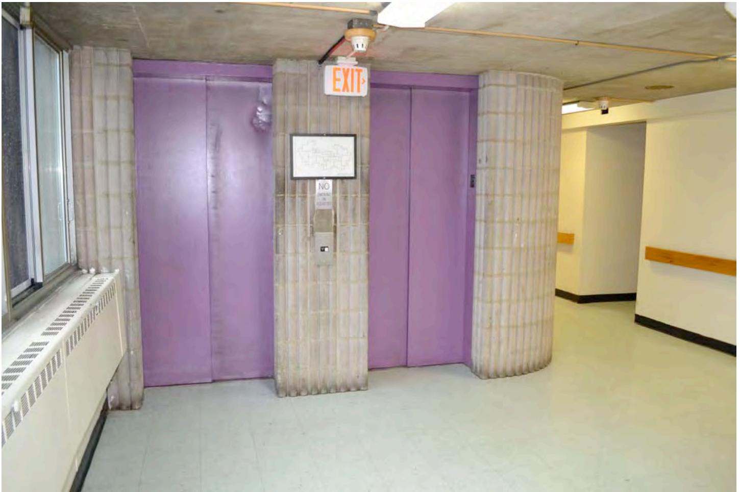
Detail of typical upper-floor elevator lobby, showing elevator, floor, wall, and ceiling details. Camera facing southeast. Photograph 13 of 19.
