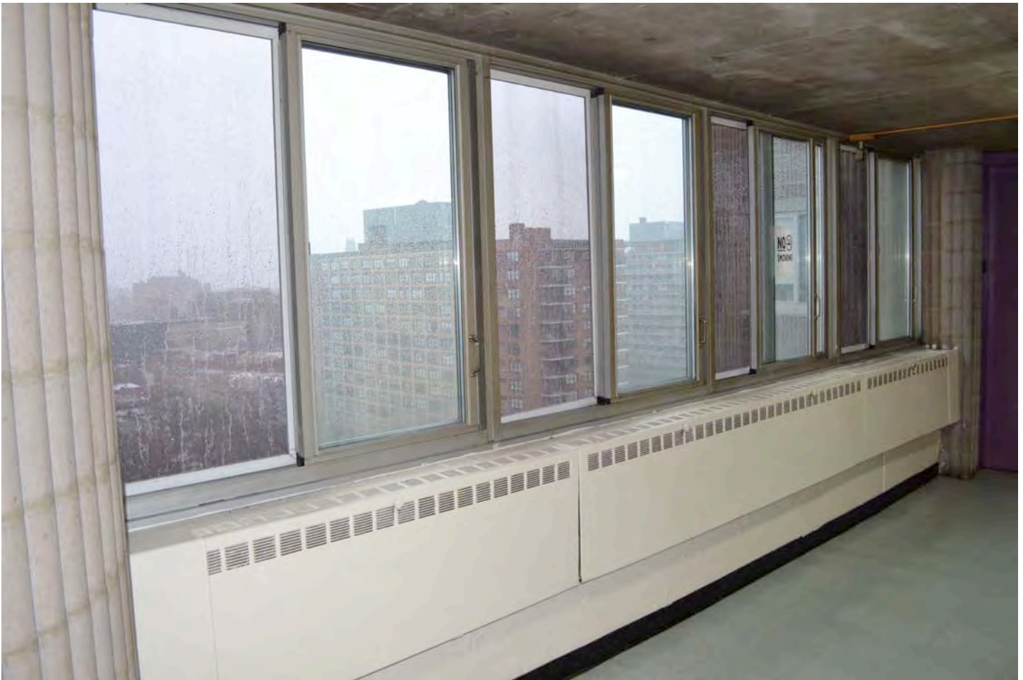
Detail of typical upper-floor elevator lobby, showing window, floor, wall, and ceiling details. Camera facing northeast. Photograph 15 of 19.
