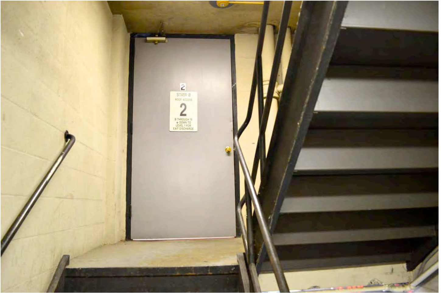
Detail of second-floor emergency stair landing, showing floor, wall, stair, rail, and ceiling details. Camera facing northwest. Photograph 12 of 19.
