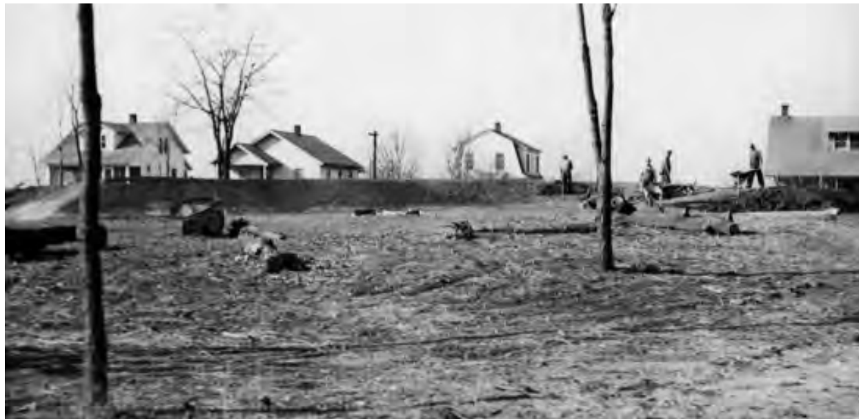
Figure 18. Workmen using hand tools to patch earthworks 1936 looking southwest. SOURCE: Courtesy of Southeast Missourian newspaper.
