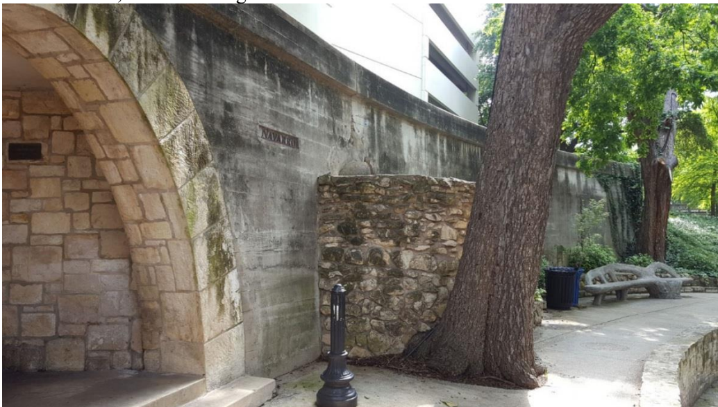
Photo 36 Block 3 (Romana Street S24 to N St. Mary's Street Bridge S26) Navarro stairs, Camera facing SW
