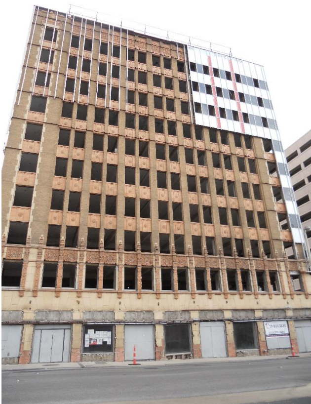
Photo 32 601 N St. Mary's, Real Estate Building (November 2017; Photo by Ann McGlone) Camera facing N
