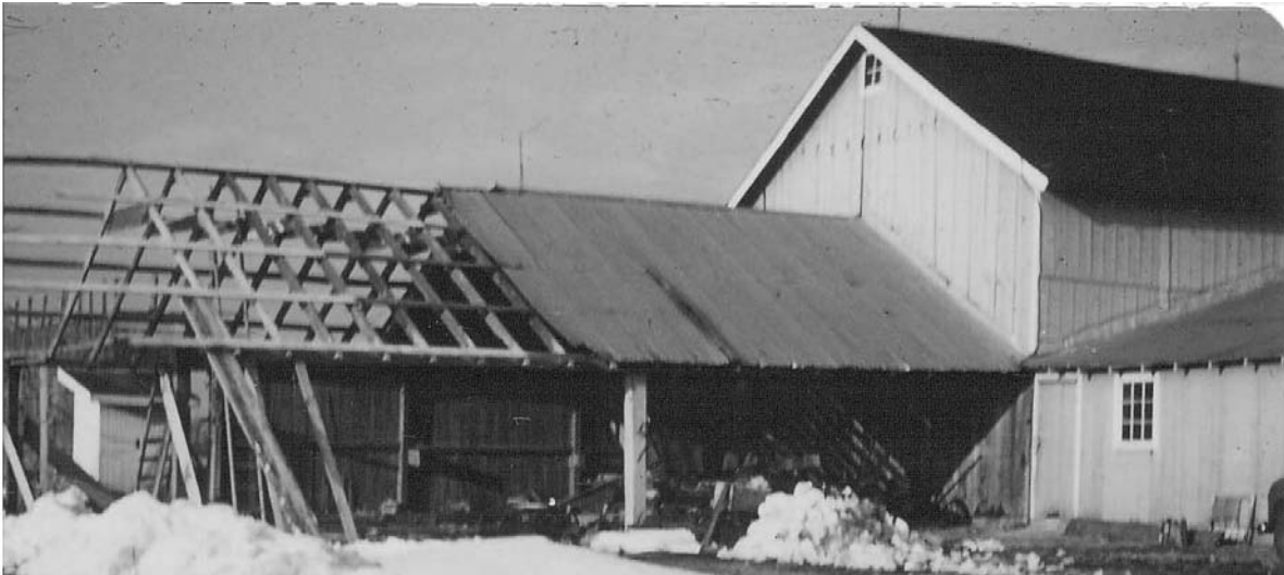
10. The rebuilding of the equipment shed after Hurricane Hazel in 1954. (Courtesy Suzanne H. Culver)
