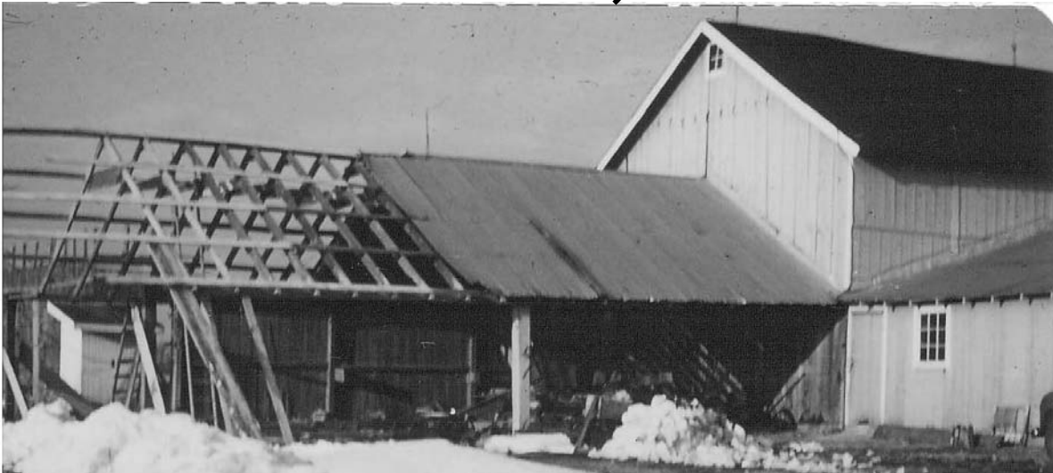
10. The rebuilding of the equipment shed after Hurricane Hazel in 1954. (Courtesy Suzanne H. Culver)
