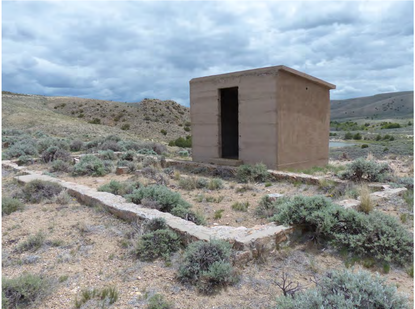
Photo #38: Engineer's Camp, Feature C (concrete foundation) and associated concrete structure Feature B, north and west elevations. Camera facing east-southeast.
