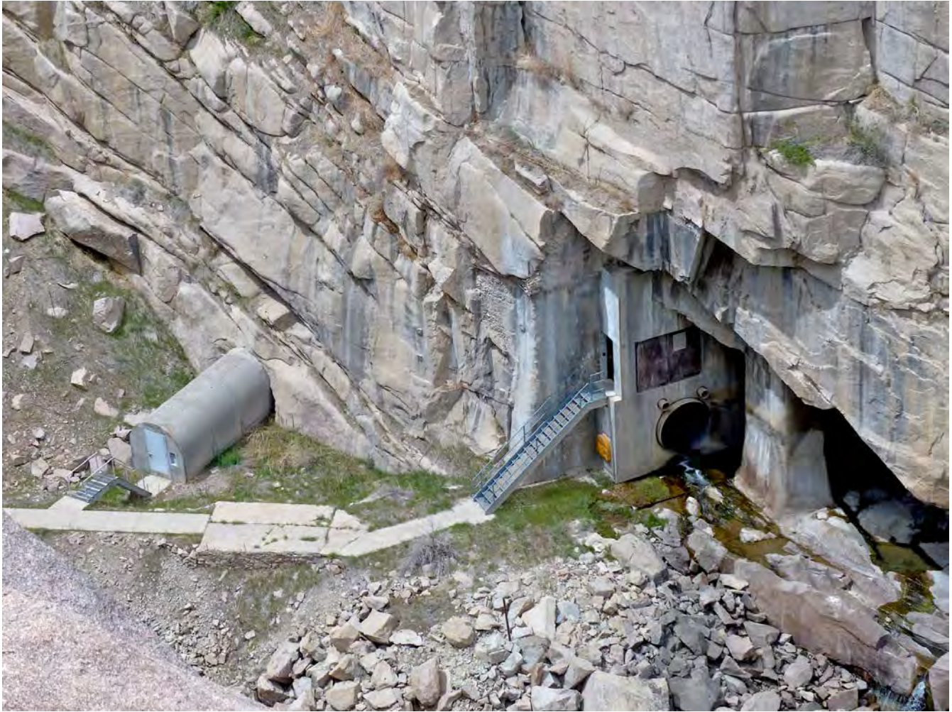
Photo #10: Canyon floor below Pathfinder Dam, north side of river, showing the access structures to the high-pressure gates (Quonset hut to left) and the river outlet works control house (right in canyon wall), and the outlet for the 60-inch Jet-Flow valve (all part of Feature E, non-contributing). Camera facing downward and northwest.
