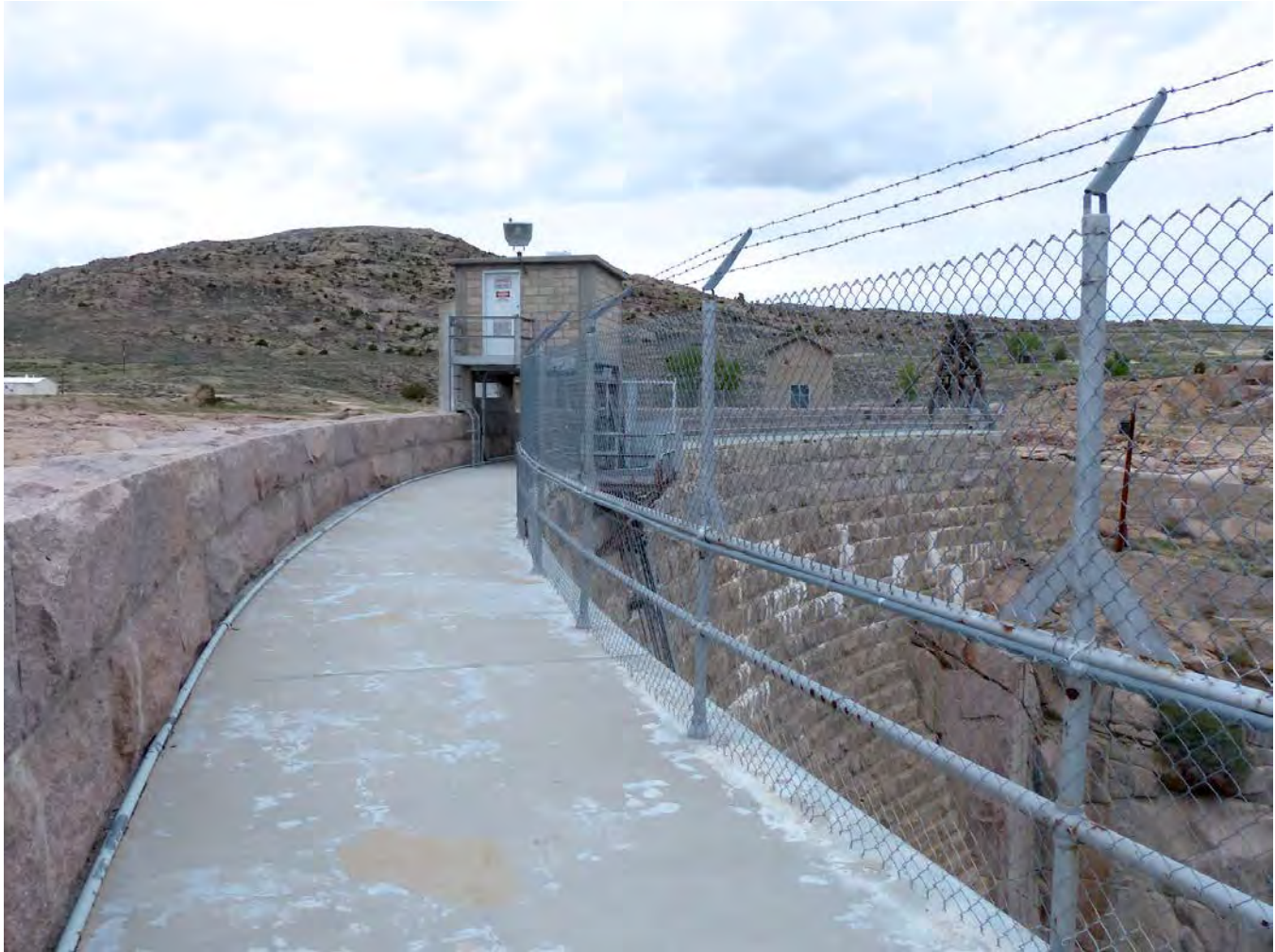
Photo #14: Pathfinder Dam crest, note safety fencing on right and parapet wall on left, and elevator machine house. Sluice Gatehouse and north cableway tower are immediately to the right of elevator machine house. Camera facing north.
