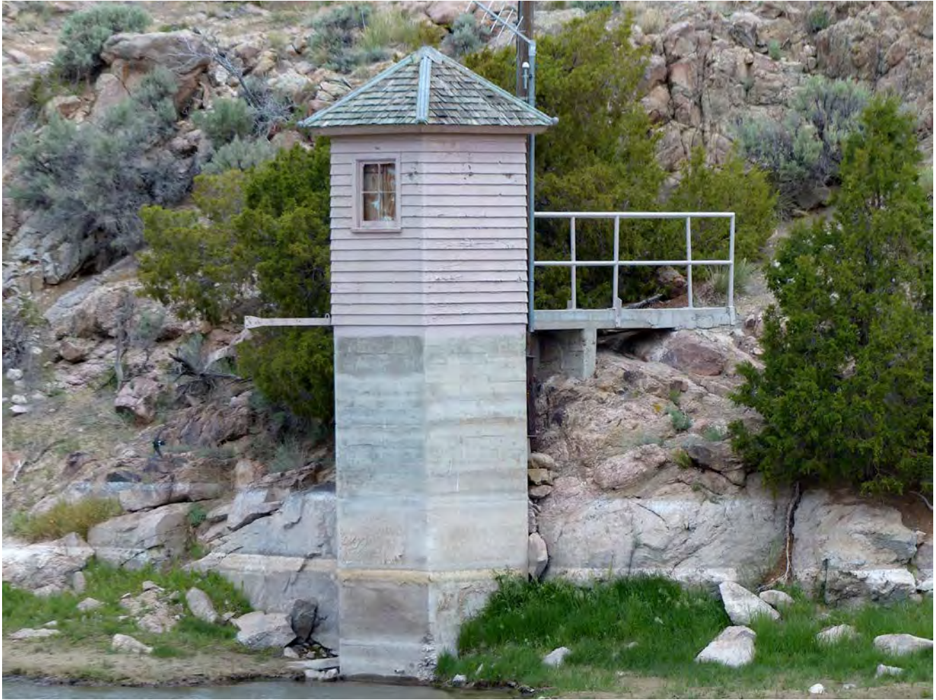
Photo #35: Stream gage station, east and south elevations. Camera facing northwest. See Photo #49 for north elevation view.
