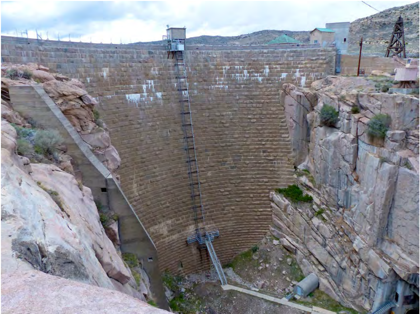
Photo #3: Pathfinder Dam, camera facing northwest. Note south access ladderway on canyon wall in the left of the photo (Feature G, contributing). Also note the elevator and associated ladder and walkways (collectively Feature B, non-contributing) leading to high-pressure gate access structure (Quonset hut) and river outlet control house in the lower right corner of the photo (both part of Feature E, non-contributing).
