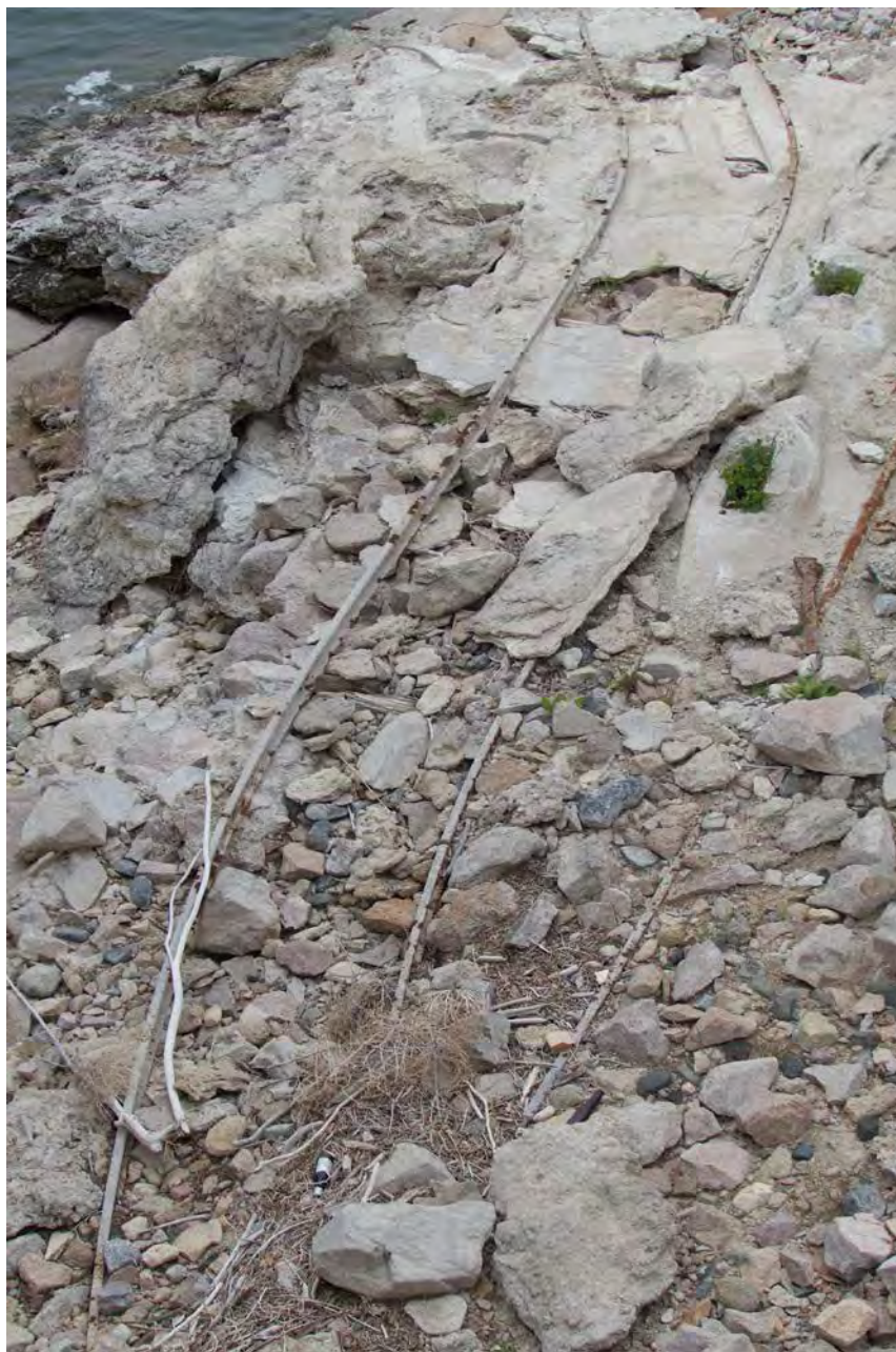
Photo #50: Last known remnants of rail system (Feature R, contributing structure) used to haul blocks from the quarries to the dam. It is located next to the dam's upstream face just below the Emergency Gatehouse. Camera facing down and to the west.
