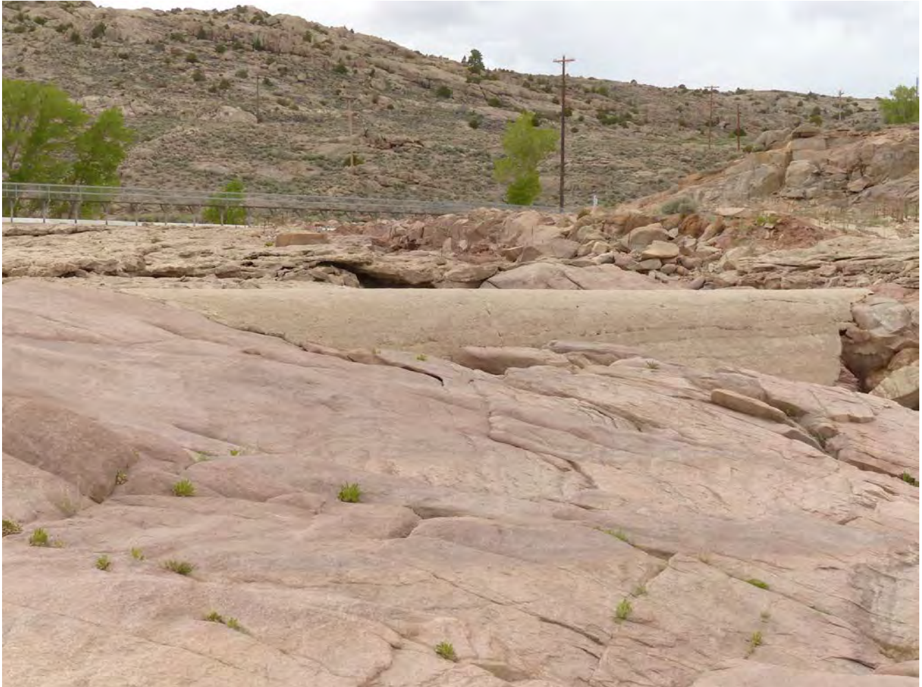
Photo #31: Remnants of the main quarry (Element 7A, non-contributing), located adjacent to the spillway. Note the concrete dike to help direct water flow. Camera facing north.
