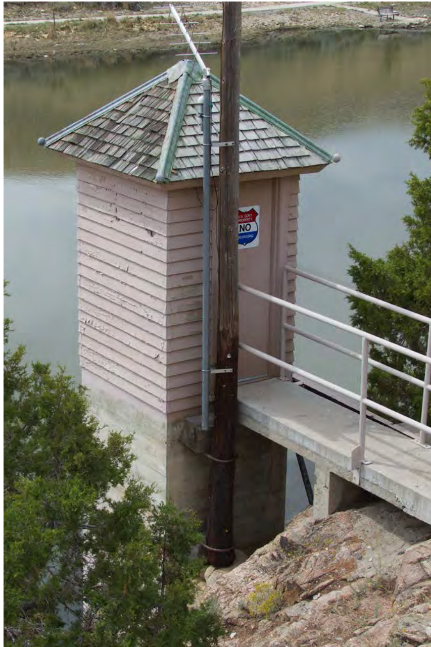
Photo #49: North and east elevations, Stream Gage Station instrument house and concrete stilling well (Element 6, contributing). Camera facing southwest.
