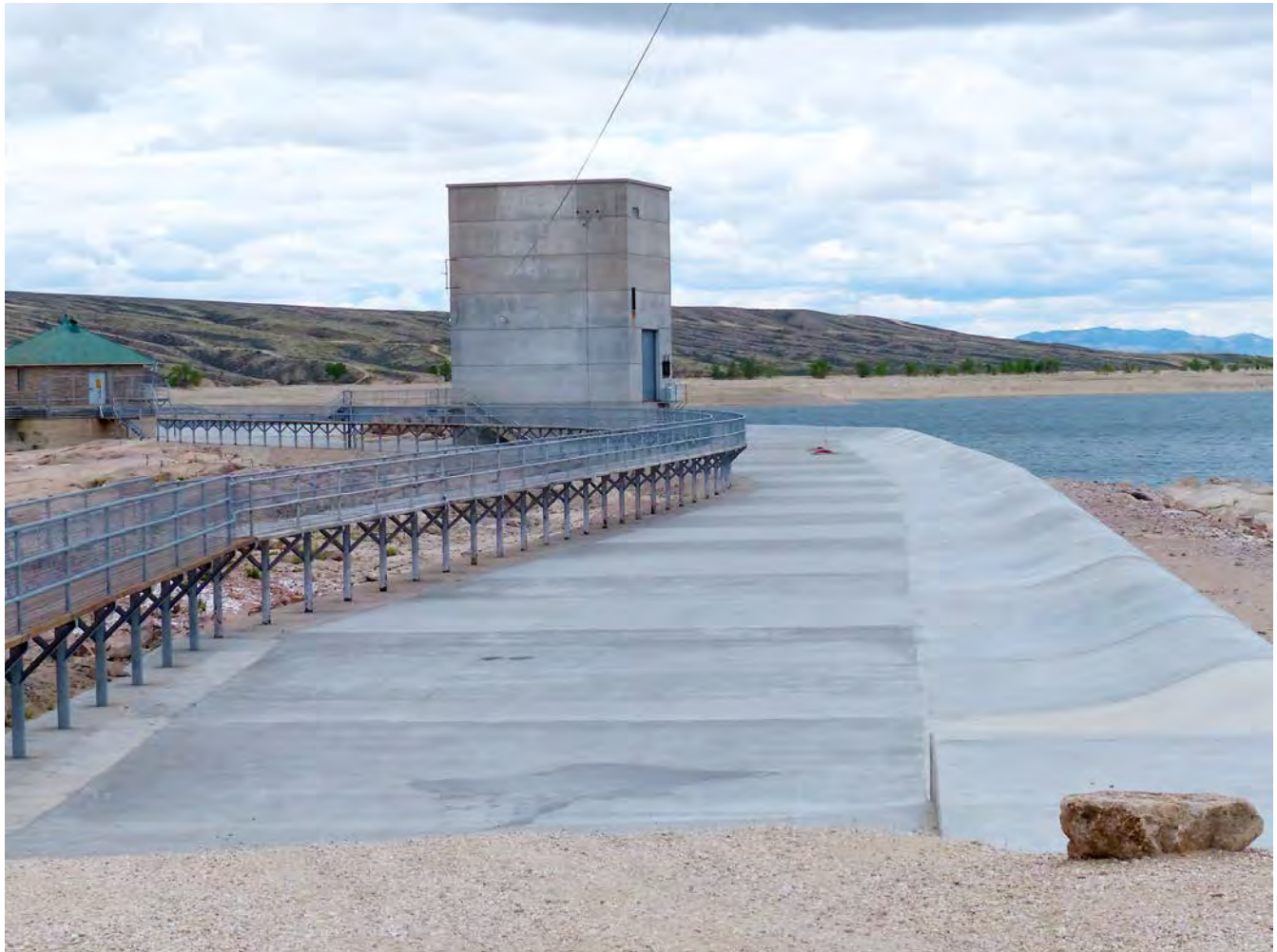
Photo #7: New spillway ogee weir and concrete apron, completed in 2012, Fremont Canyon Fixed Wheel Gatehouse, and Emergency Gatehouse. Camera facing south.
