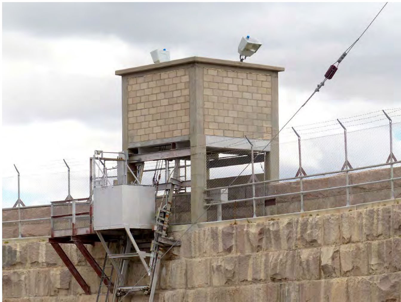
Photo #12: Elevator machine hoist house and Kimball elevator (Feature B, non-contributing). Camera facing southwest.
