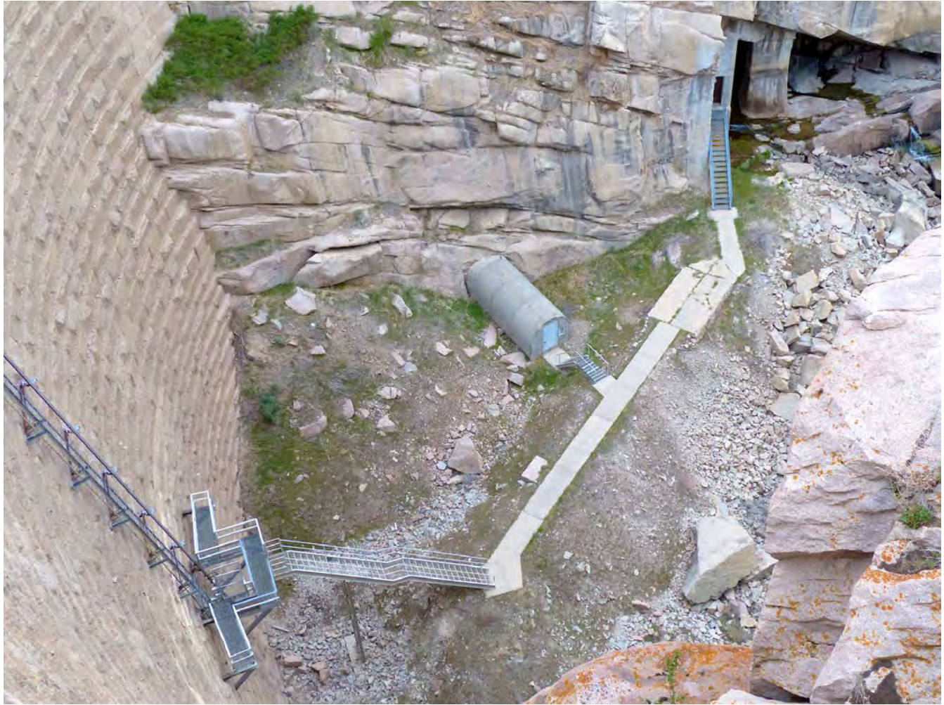
Photo #11: View from above of (from left) the dam's downstream face, the elevator track, walkway, and the high-pressure gate control (Quonset hut) access structure. Camera facing down and northeast.
