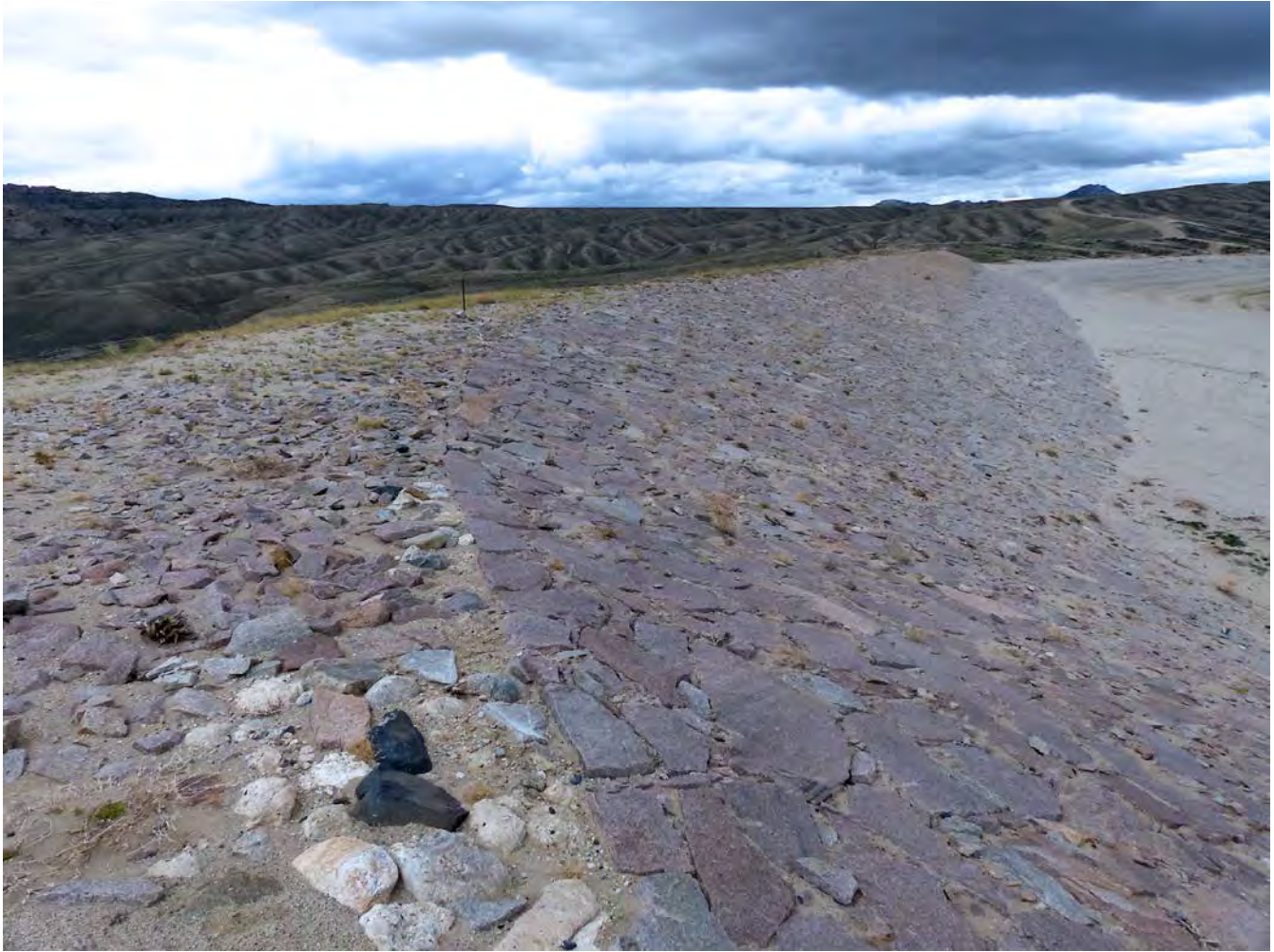
Photo #21: Pathfinder Dike (Element 2, contributing). Note hand placed granite rock protective facing on the upstream (right) side of the dike. The rubble rock visible on the downstream face is part of the earthen/rock matrix of the dike embankment. See historic photo #20 showing placement of the protective rock in 1910. Camera facing south from north end of the dike.
