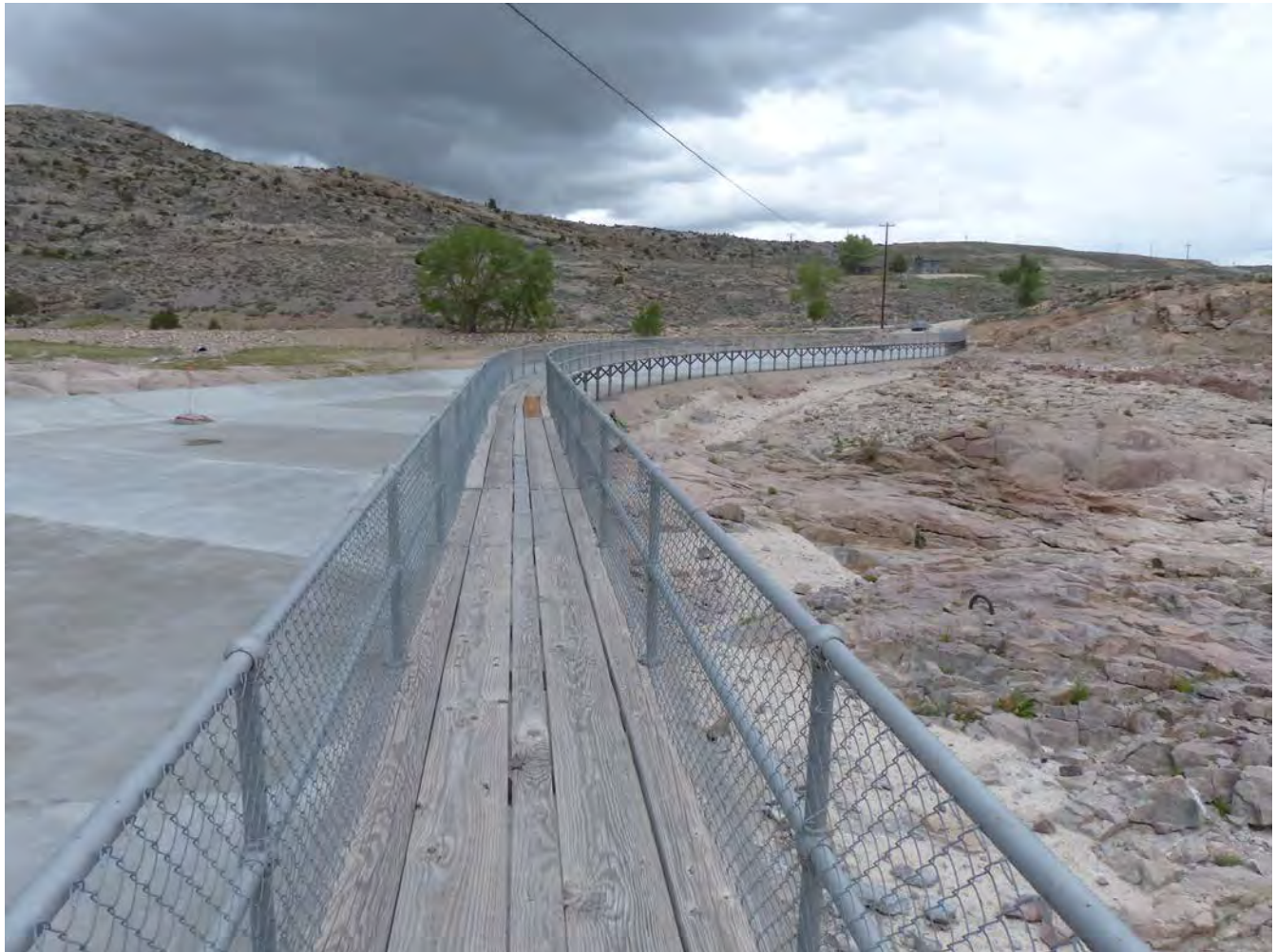
Photo #32: New spillway concrete ogee weir and apron (left, Feature J, non-contributing), facility access walkway (center, Feature I, non-contributing), and upper end of natural section of Pathfinder spillway (right, Feature H, contributing). Note the U-bolt set into the spillway bedrock. Camera facing north.
