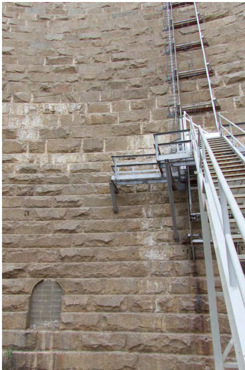
Photo #46: Stonework detail and plugged access gallery, downstream face Pathfinder Dam. Camera facing west.
