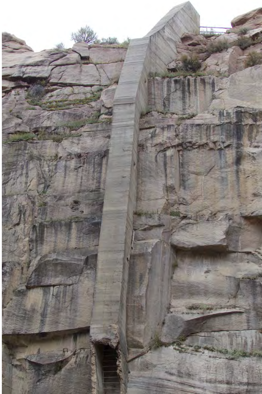
Photo #45: Abandoned concrete access ladderway (Feature G, contributing) from canyon floor. Note rebar used as ladder rungs. Camera facing south.
