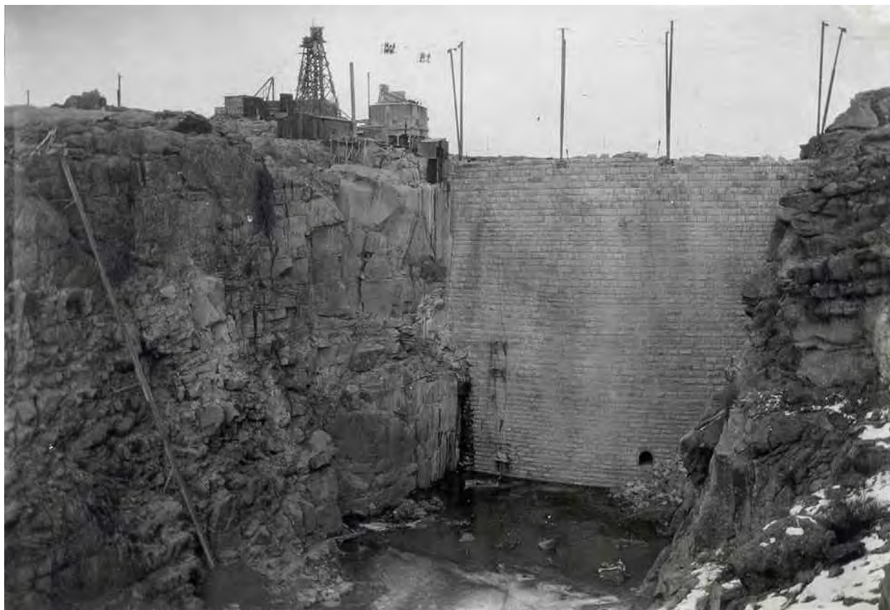
Historic Photo #13: 1908, Pathfinder Dam upstream face. North towers of original two cableway systems shown. Note exposed access ladder on left hand side of canyon, precursor to the enclosed ladderway built a few years later. Emergency Gatehouse under construction (structure immediately next to dam).
