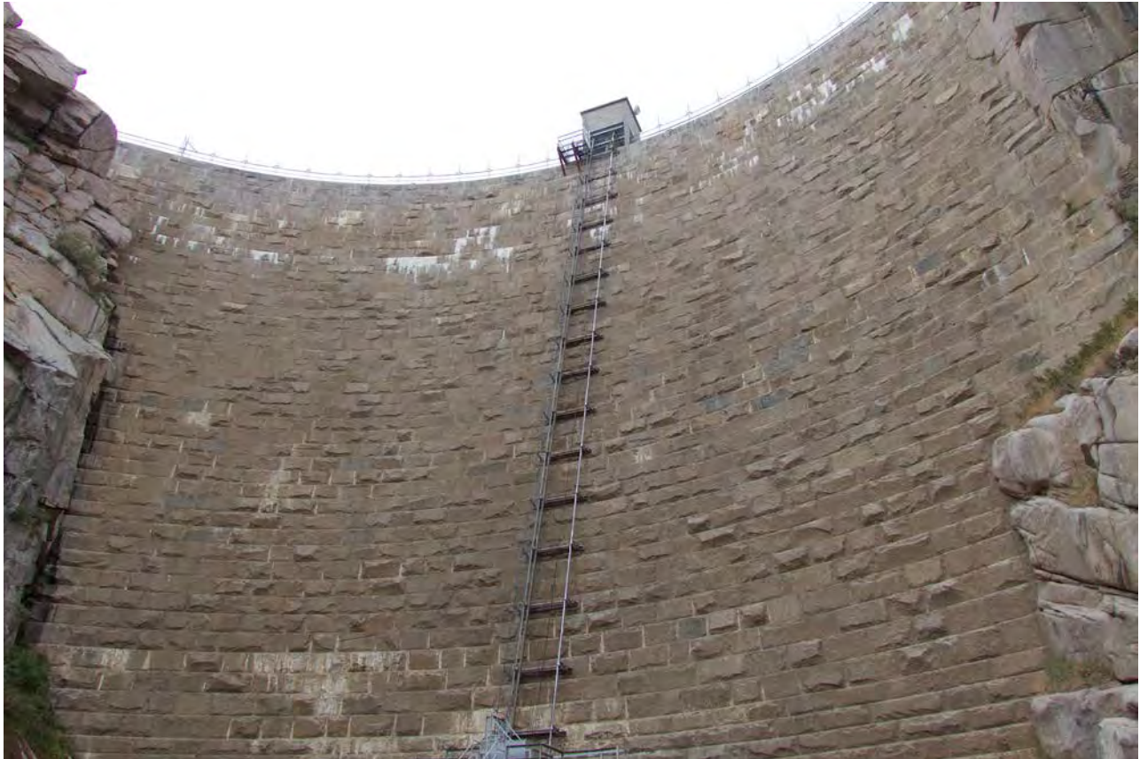
Photo #44: Upstream face of Pathfinder Dam from canyon floor. Camera facing west.
