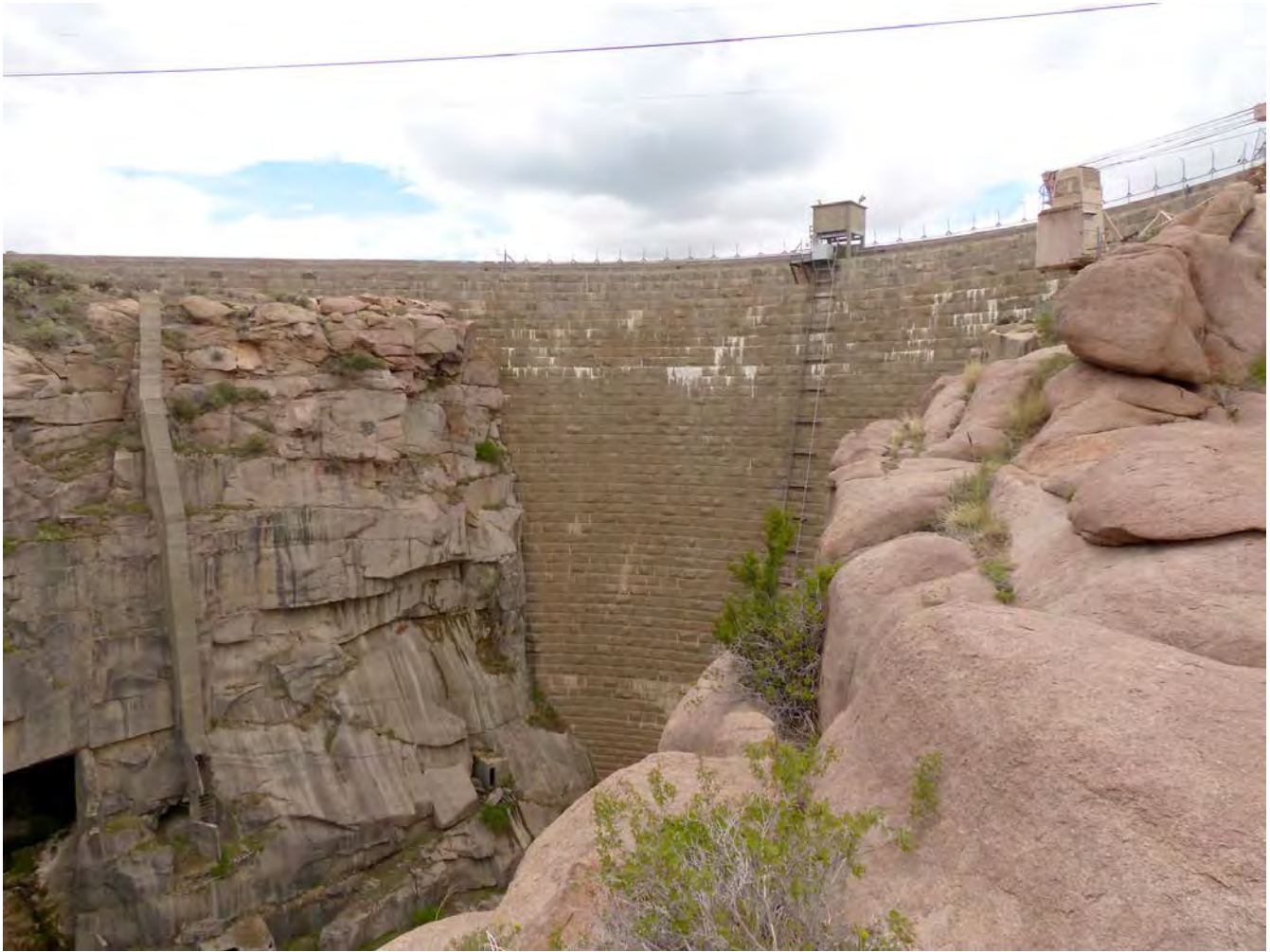
Photo #4: Pathfinder Dam, south access ladderway (Feature G, contributing), and south tunnel outlet and auxiliary tunnel balanced valve control house (both elements of Feature F, non-contributing). The south tunnel outlet is the large opening visible to lower left of the ladderway; the value house is the small structure in the rock face to the right of the ladderway. Camera facing southwest.
