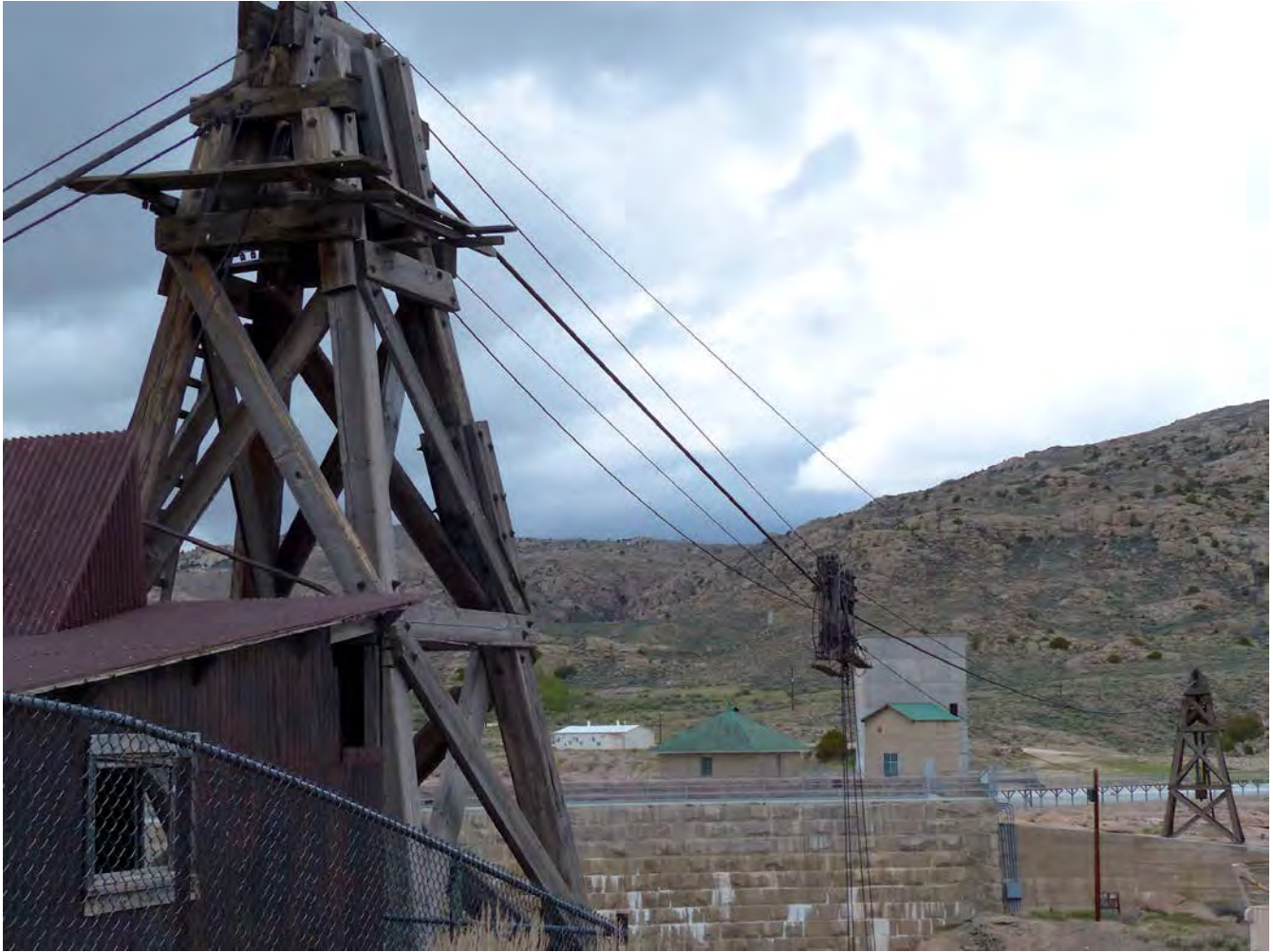
Photo #20: Long view of 1920 cableway system. From the left, cableway powerhouse, south tower, carriage cable and bucket hook system, and north tower. (Features M and N, contributing). Camera facing northwest.
