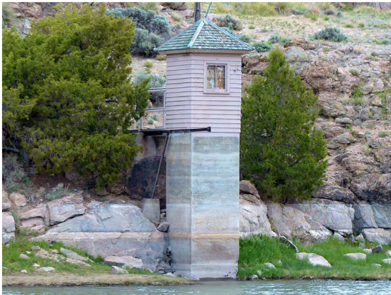
Photo #34: Stream gage station, south and west elevations (Element 6, contributing). Camera facing northeast.
