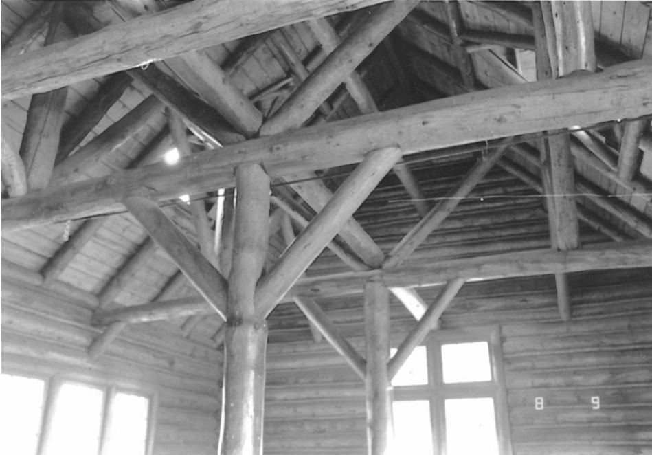
Photo H3. Interior view of roof trusses, dated 8/9/1993. On file with the Office of Archaeology and Historic Preservation, History Colorado
