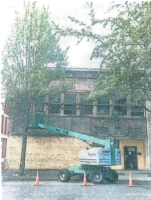
The original windows at 440 State St. have been uncovered in the process of its historic preservation through a state grant. SPECIAL TO THE STATESMAN JOURNAL
