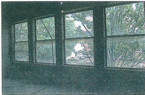
State preservation officials determined the windows in the building at 440 State St. can be restored given their condition. ELIDA S. PEREZ / STATESMAN JOURNAL
