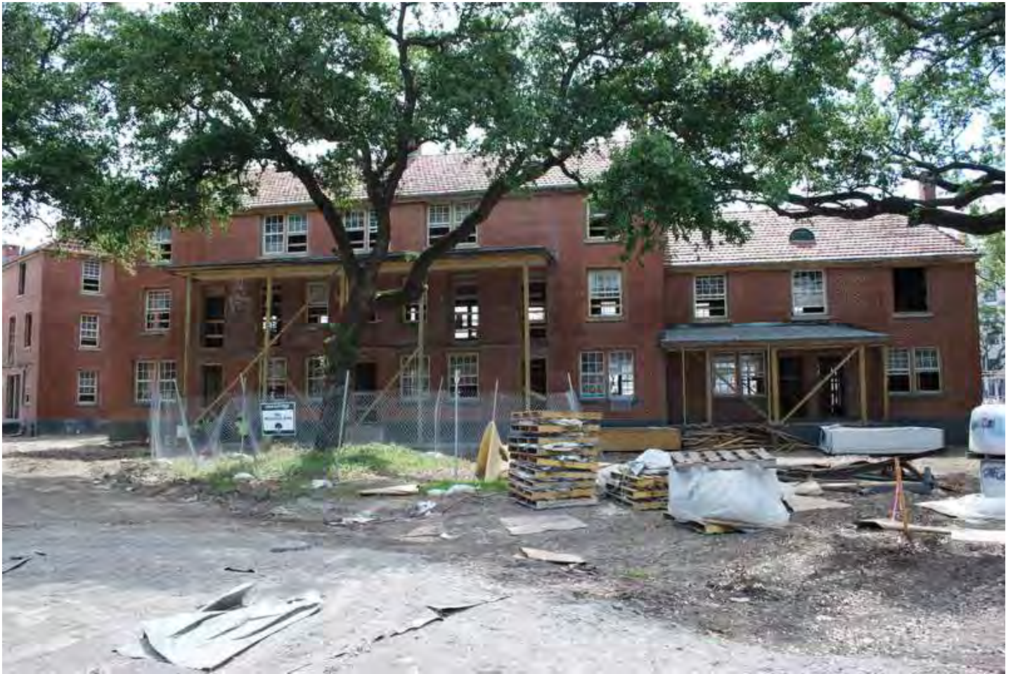
Figure 12. Building #69. Photograph dated: May 27, 2014. On file, R. Christopher Goodwin & Association, Inc., New Orleans.
