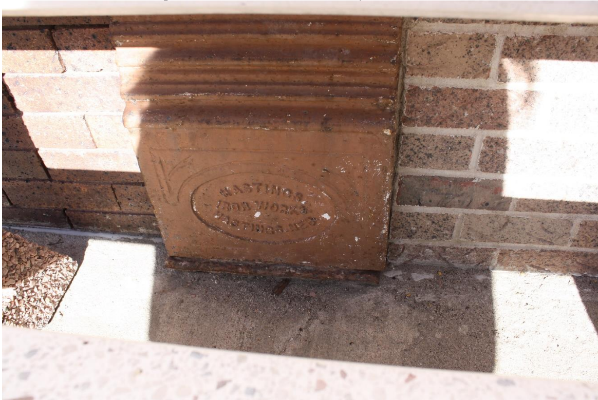
Hastings Iron Works column base at Stein Building on West 2nd Street.
